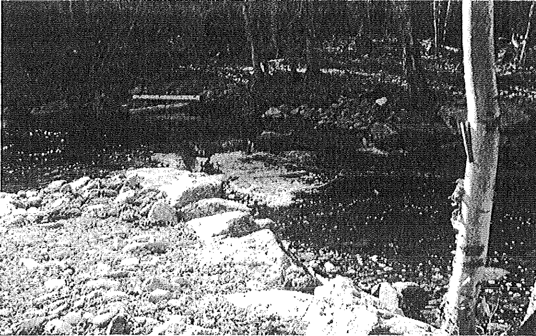
Rock weir No. 2, Lower Project, October 2007, two months after construction. The river-left log deflector of the lower-most pair (which suffered ice damage) was removed to construct this weir.
