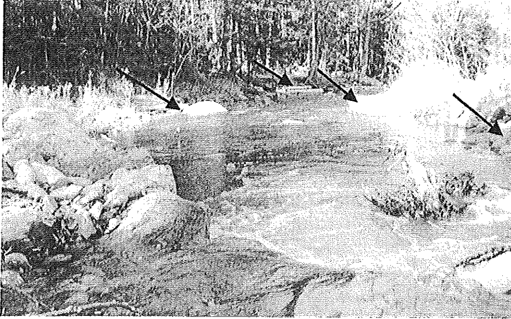
Transect 12 looking downstream after construction of rock weir no. 1, October 2007. Wing of rock weir is at left; pool and root wad visible immediately downstream of weir. Four log deflectors (highlighted by arrows) are visible downstream. The left log deflector of the second pair was removed in order to construct this weir.
