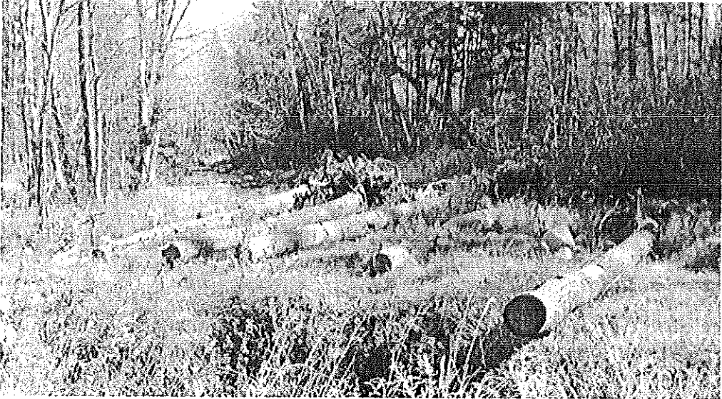
Cabled logs with attached root wads, Middle Project, east shore, October 2007, 14 months after construction. Little sediment has been trapped by these logs to date.
