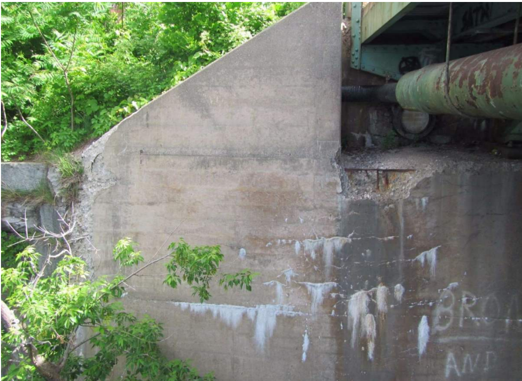
Photo 26: Abutment 2 (Lewiston end) concrete deterioration
