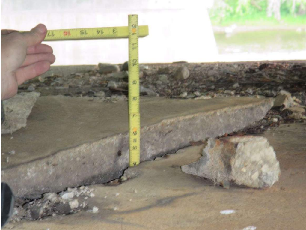
Photo 33: Pier 2 pier cap cracking and soft concrete
