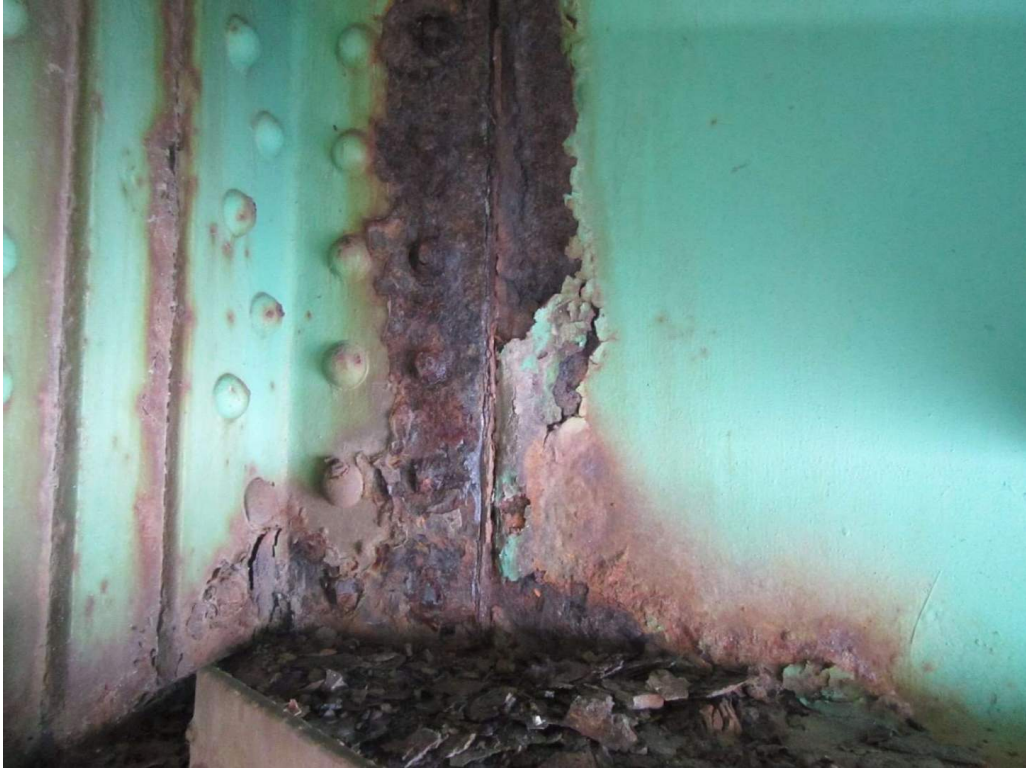
Photo 21: Floorbeam connection with deteriorated rivets
