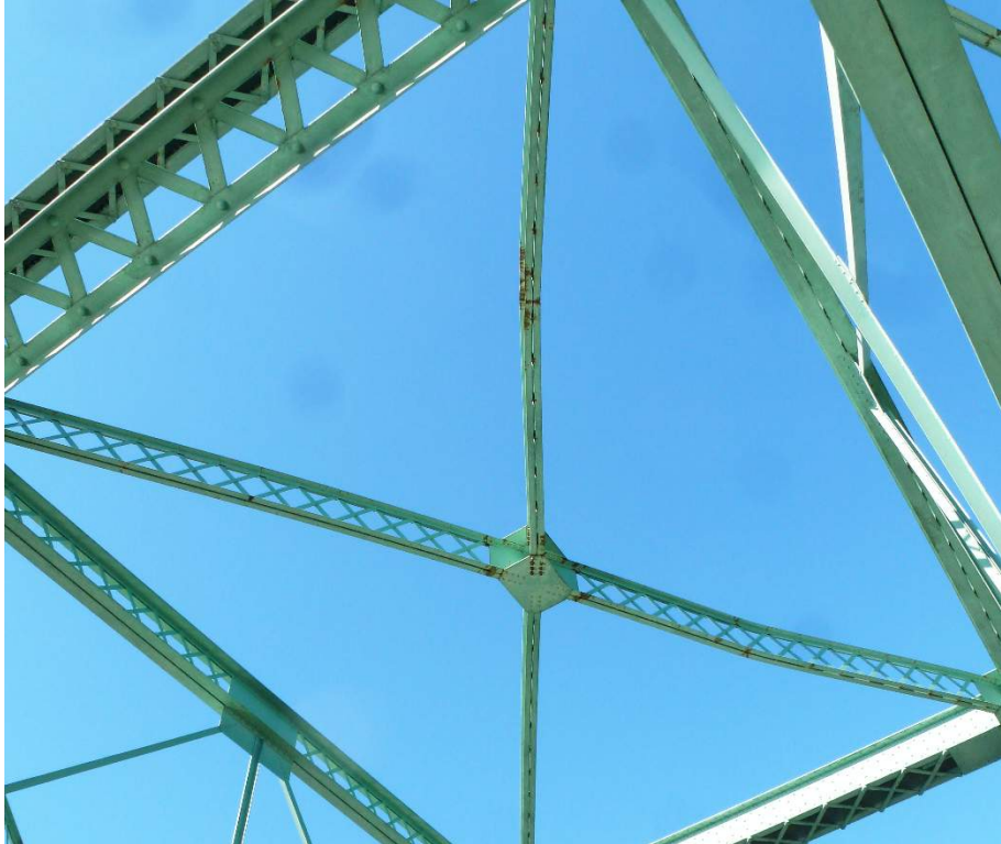
Photo 23: Bent top diagonals (Span 3 truss)
