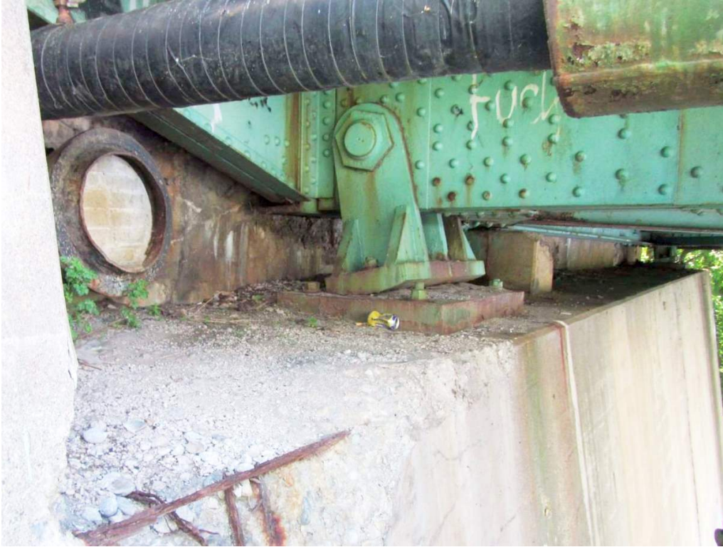
Photo 27: Abutment 2 (Lewiston end) bearings rocked out of plumb (high temperature of 73 degrees on the day this was taken)
