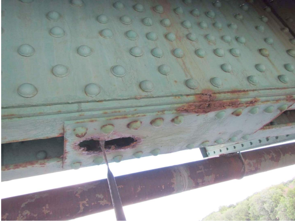
Photo 19: Hole through bottom chord bottom flange splice plate (downstream side of truss, near the end of Span 2)
