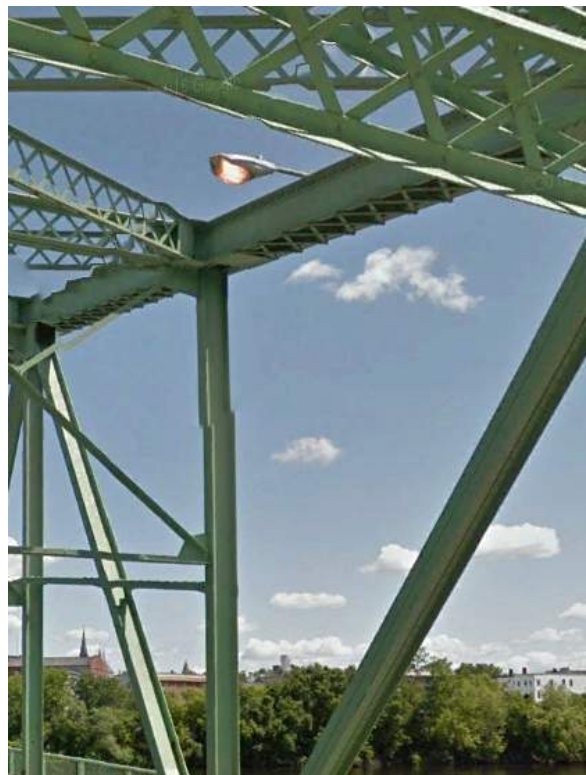
Photo 34: Existing bridge lighting (From Google Streetview)
