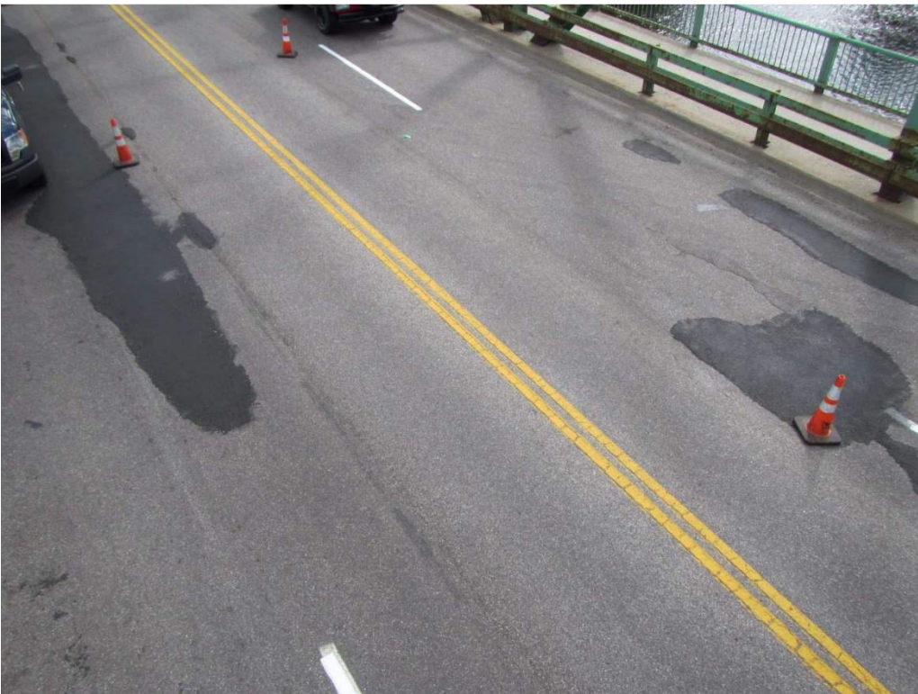
Photo 10: Wearing surface patches
