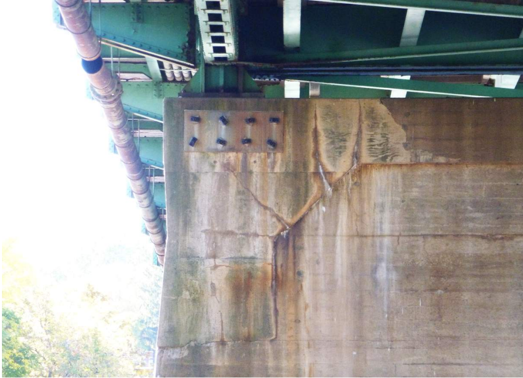
Photo 31: Pier 2 pier cap close-up showing 1995 failure location and deteriorating repair
