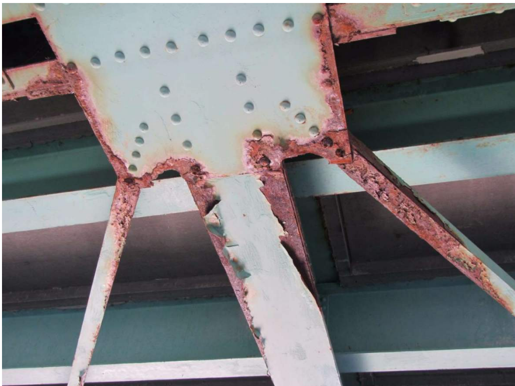
Photo 24: Bottom lateral bracing connection plate (worst case section loss)
