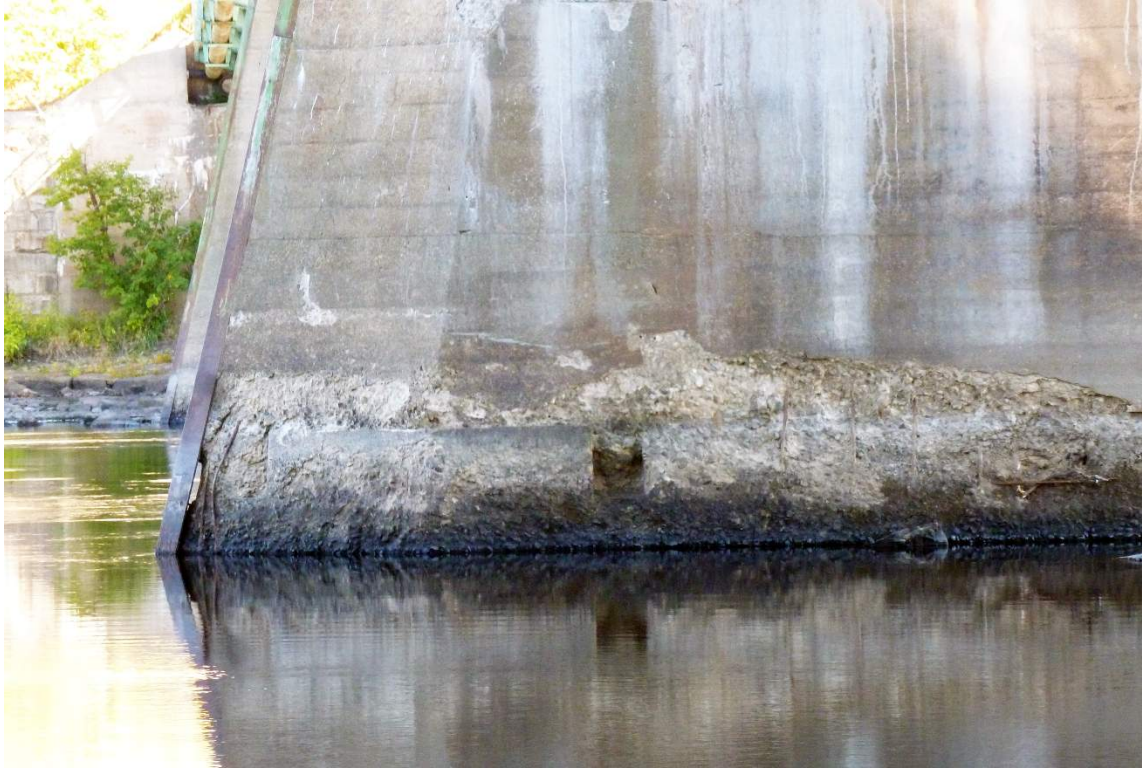
Photo 29: Pier 1 water line deterioration
