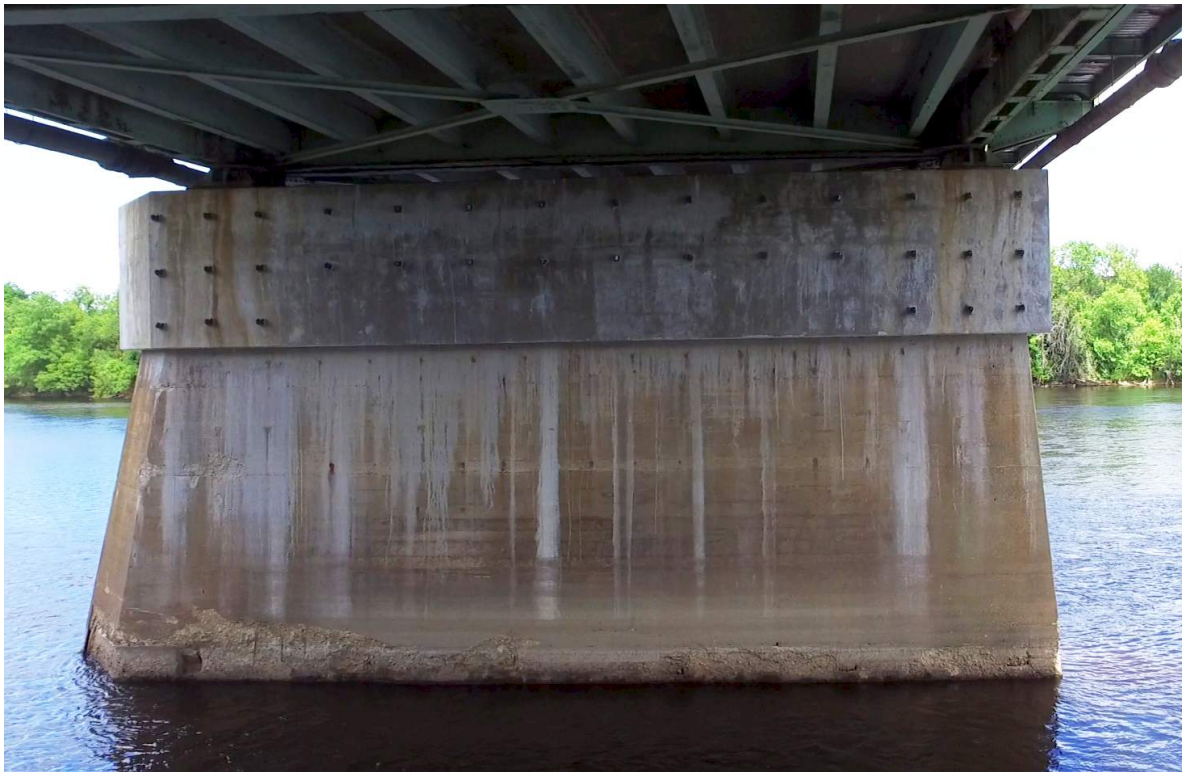
Photo 28: Pier 1 elevation view showing 2014 pier cap repair and deterioration at water line
