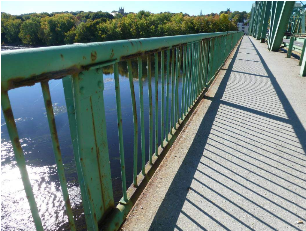
Photo 22: Sidewalk railing showing bent ballusters
