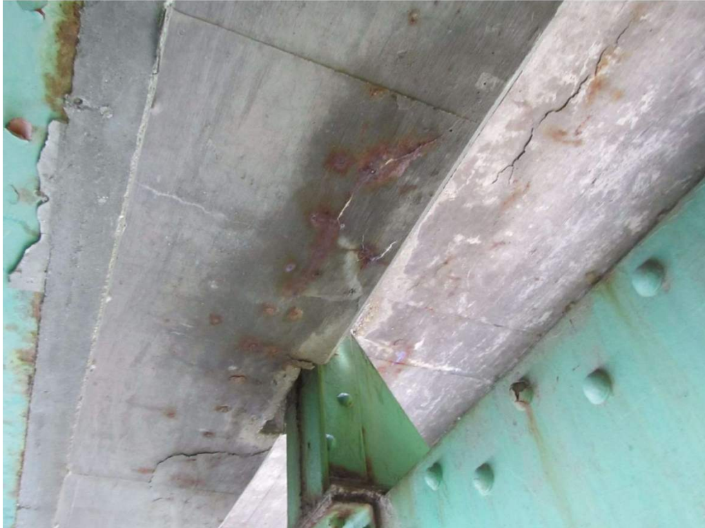
Photo 11: Deck delaminations (isolated areas – this area is around a deck penetration for a traffic rail post)
