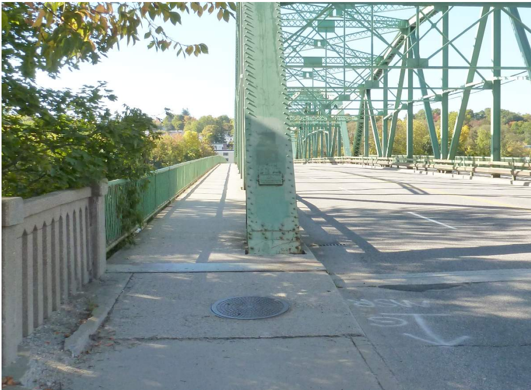
Photo 12: Unprotected end of truss (typical for all corners; this view from Lewiston approach)
