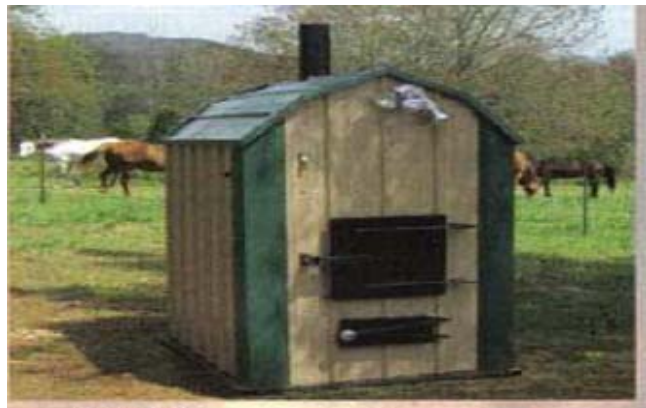
Figure 2. Typical OWHH installation.
