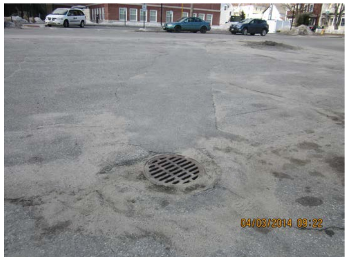
View of the catch basin at the western parking lot at the Site.
