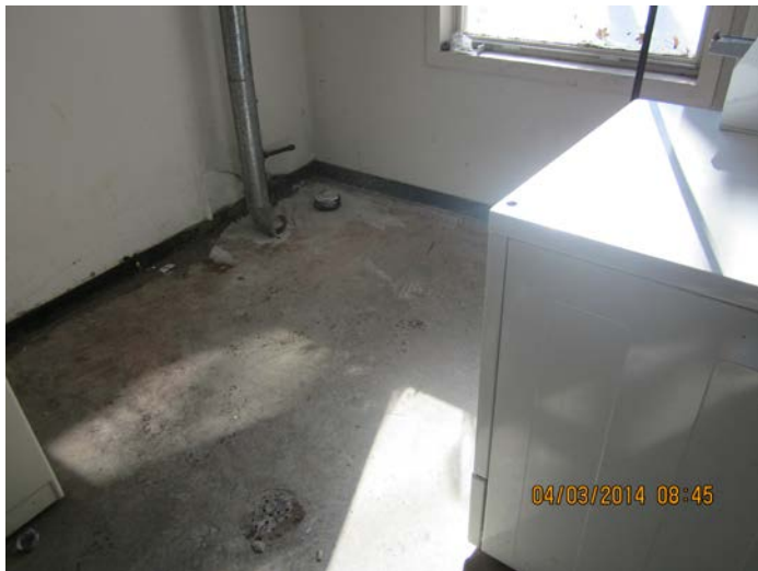
View of the laundry room in the building. Note the floor drain in the center of the room.
