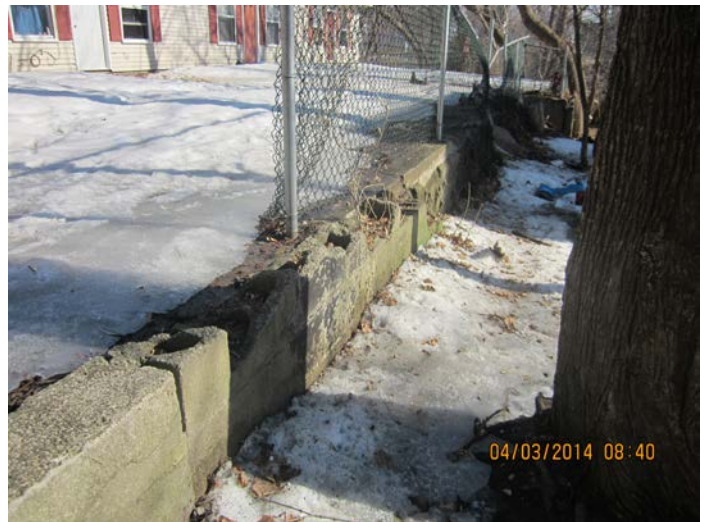
View of the remaining concrete foundations of the former Beal's Linen and Malo Cleaners buildings along the southern property boundary.
