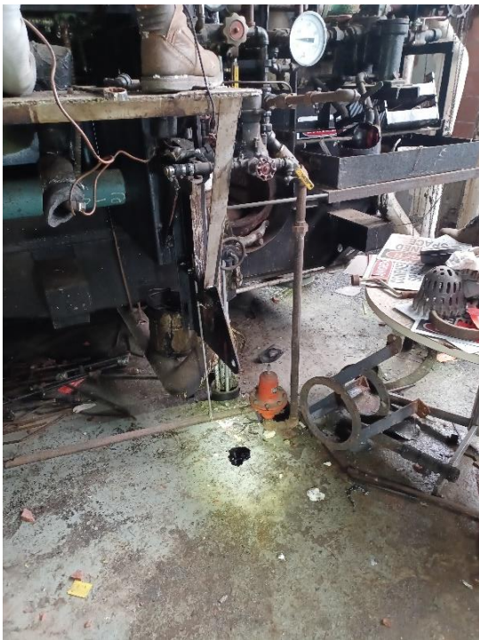
Photo 29: #6 Oil Release From Equipment at Main Entrance in Units 1 & 2
