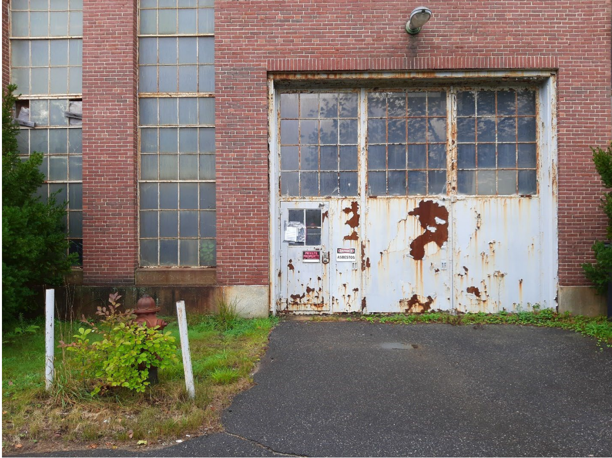
Photo 3: Warrant posted on door to the Power House Building at the Site. Door was centrally located on the River side of building. Photo by Chris Redmond, MEDEP
