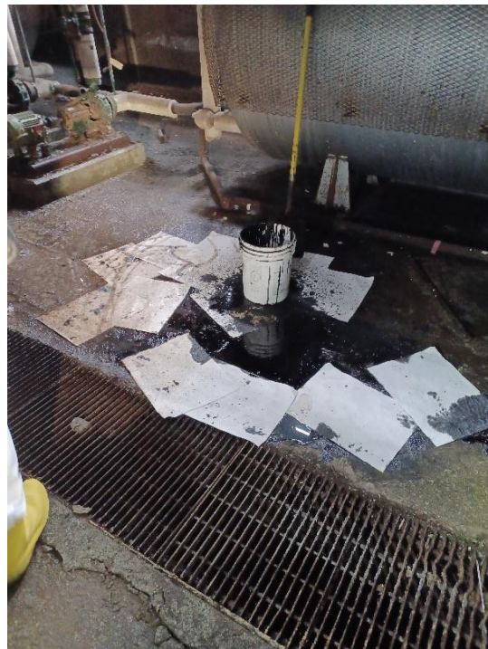
Photo 30: #6 Oil Release in Units 1 & 2 Leaking From Lockers on Mezzanine Above
