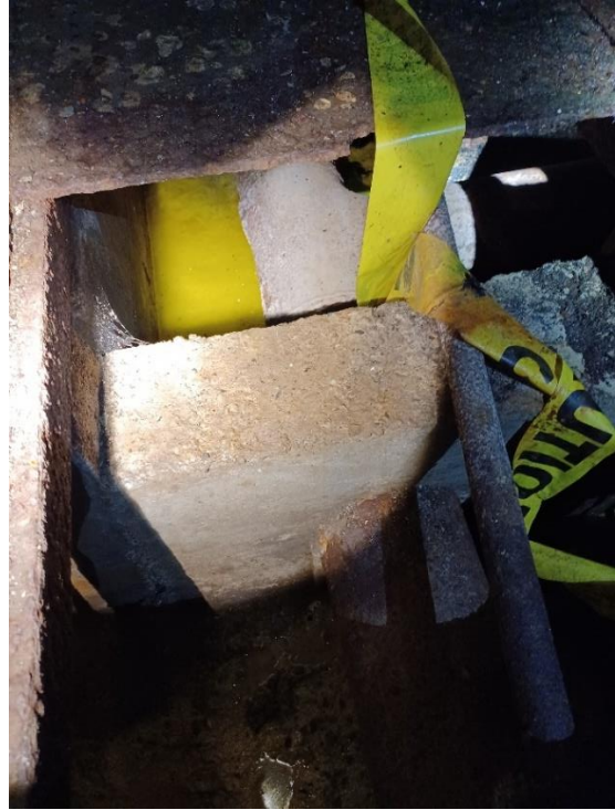
Photo 32: Unknown Yellow Substance in Units 1 & 2 Floor Bays Around Piping Banks. Not Sampled.
