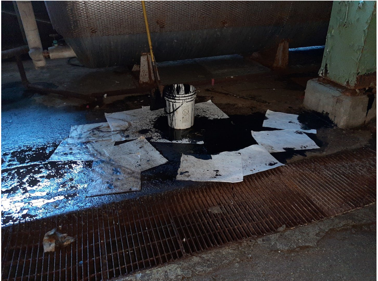
Photo 7: “Hazardous Substance” sample location. Thick, viscous oily substance suspected to be No. 6 oil. Sample collected from bucket and floor near bucket. Material was leaking from overhead pipe. Trench drain covered in grated metal in foreground. Photo by Chris Redmond.
