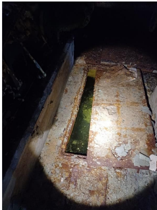
Photo 33: Unknown Yellow Substance in Units 1 & 2 Floor Bays Around Piping Banks. Not Sampled.
