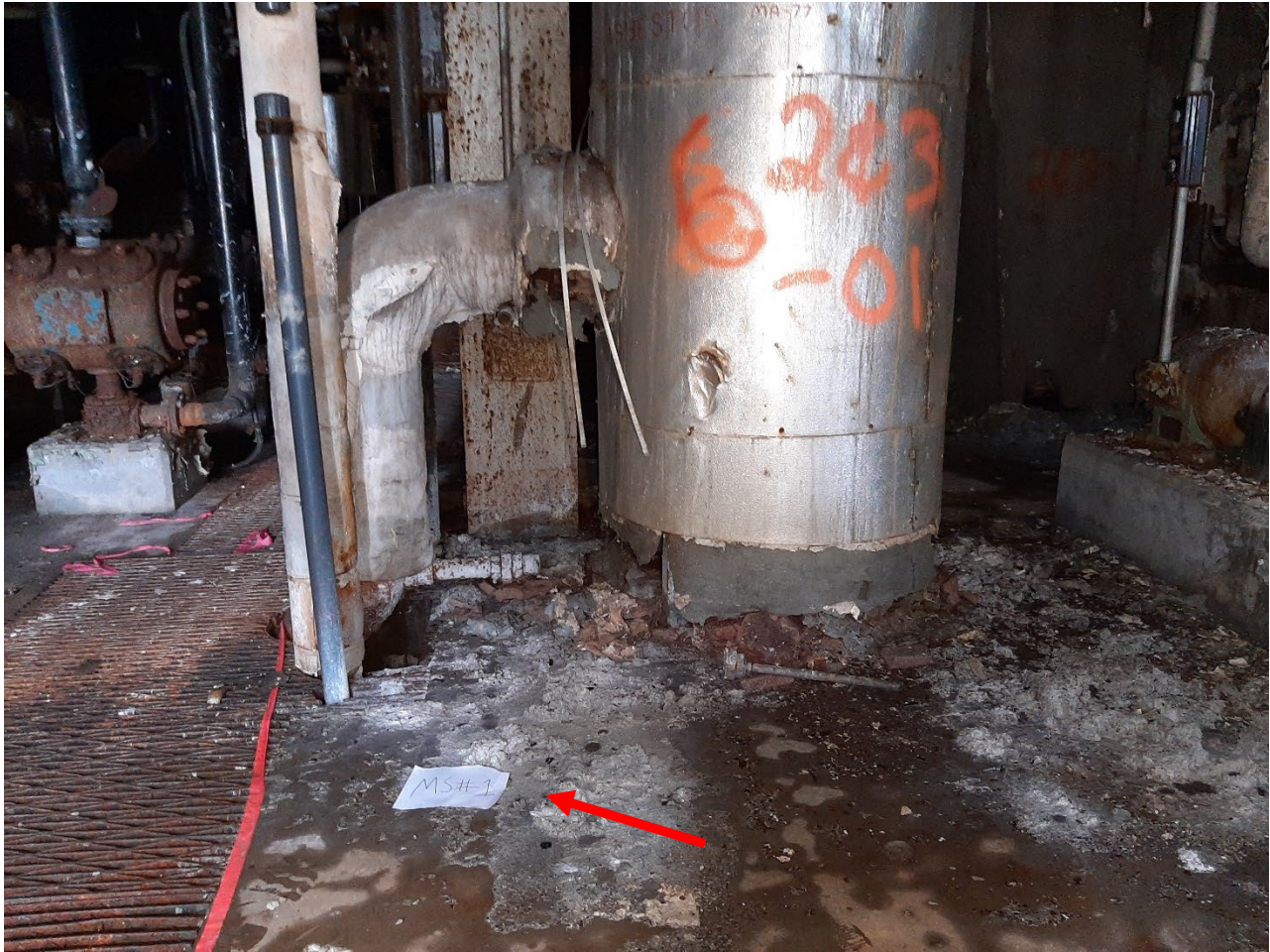
Photo 1: MS#1 location shown by red arrow. Trench drain covered in grated metal on left of photo. Photo by Chris Redmond.
