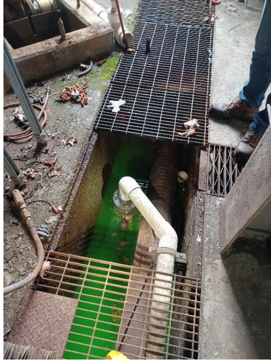
Photo 24: Tracer Dye in EF-07 Floor Trench in Unit 5
