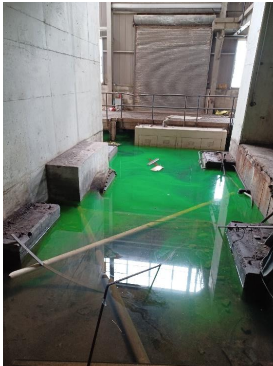
Photo 25: Tracer Dye in Unit 5 Vault Where EF-08 & SD-419 Samples Were Collected
