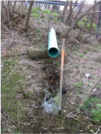
This outfall, though in poor condition because it is cantilevered, provides a good opportunity for a clean catch of its discharge.
