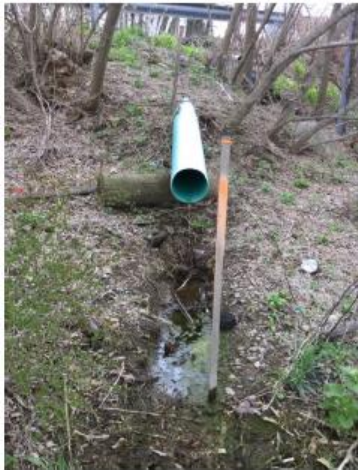
This outfall, though in poor condition because it is cantilevered, provides a good opportunity for a clean catch of its discharge.
