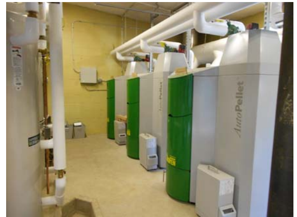
Carrabec High School pellet boilers (Photo courtesy of Cordjia Capital Projects Group)
