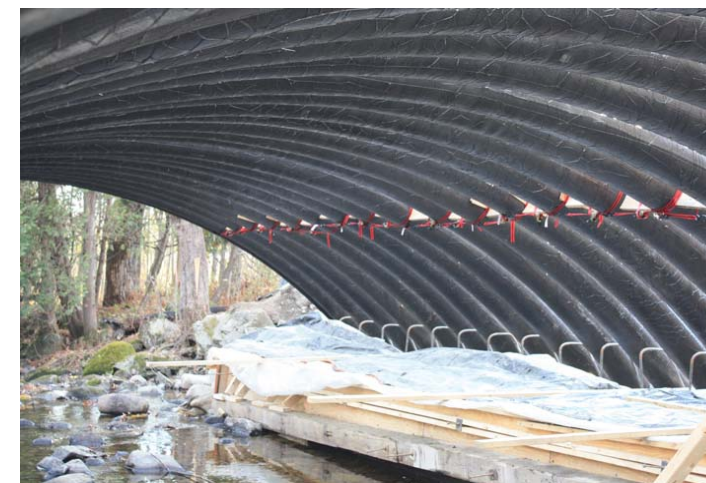
Underside of Neal Bridge, first field application of Bridge in a Backpack
