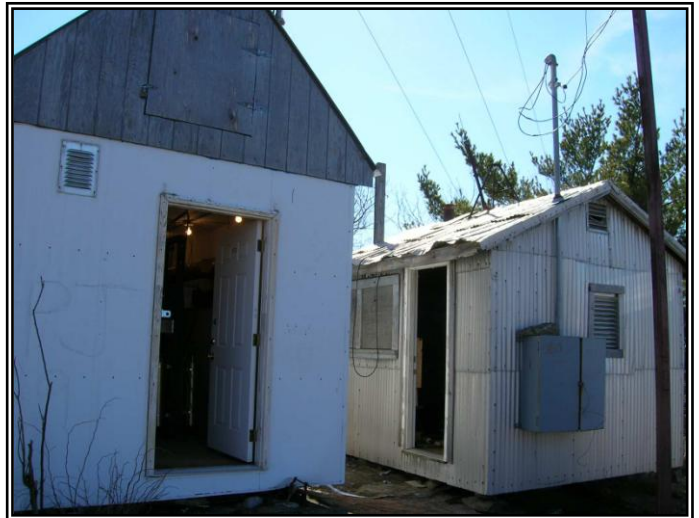
Figure 2: Old radio shelters scheduled for replacement with MSCommNet project.
