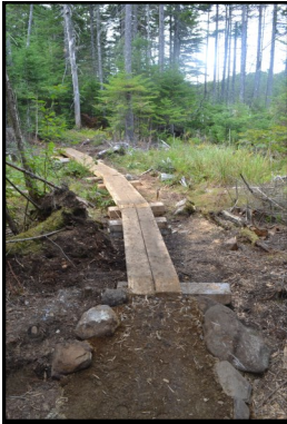
Milled-cedar bog-bridging near Cranberry Pond. These structures provide a bike-able (albeit narrow) surface over wet soils
