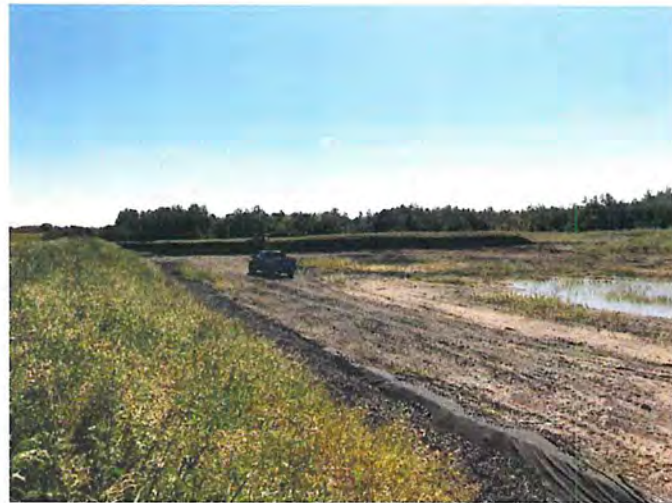
Dolby III Temporary Cell for Lagoon Waste
