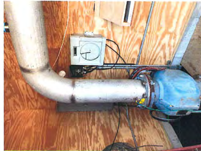
Leachate Flow Meter
