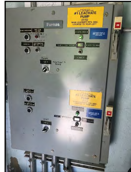
Leachate Pump Control Panel
