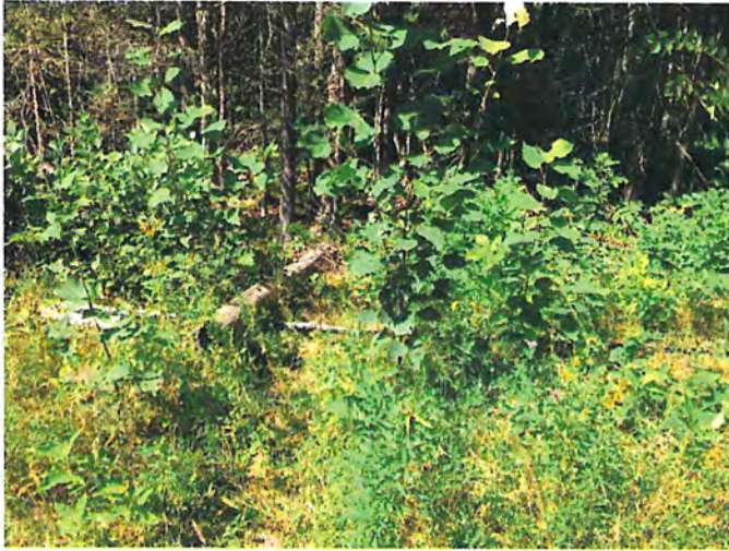
Communication Damage- Leachate Pipeline Pole
