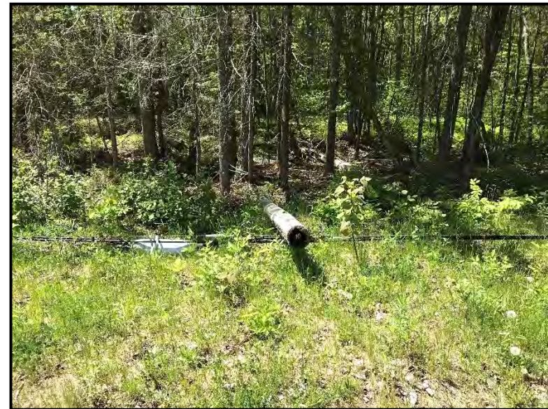
Transition Station Power Line
