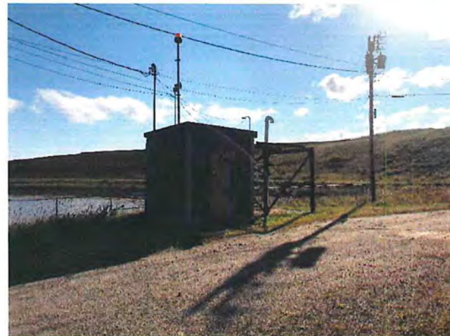
Leachate Pump Station
