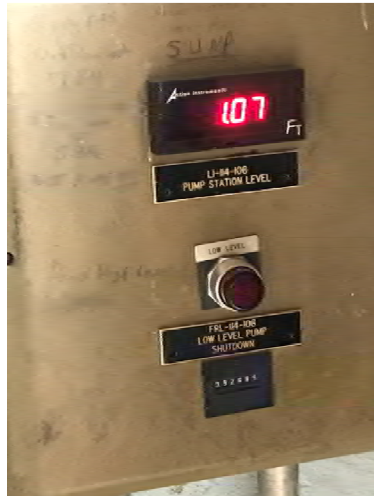
Leachate Pond Pump Station Level Display
