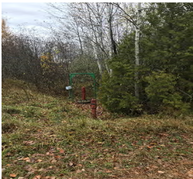
Leachate Pond Underdrain Pump Station
