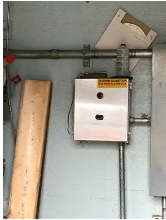
Underdrain Pump Run-Time Meter
