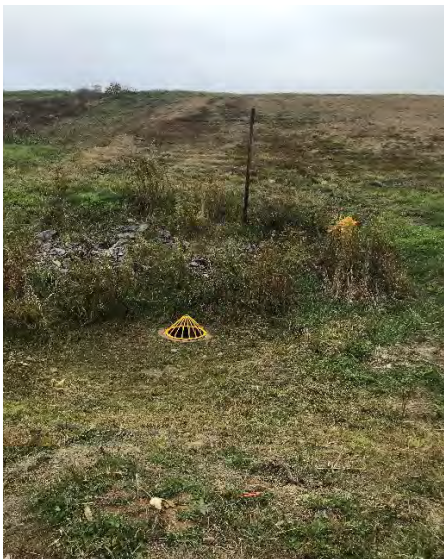
Dolby III Stormwater Inlet
