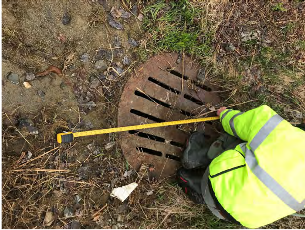
Dolby III Catch Basin (Item 10)
