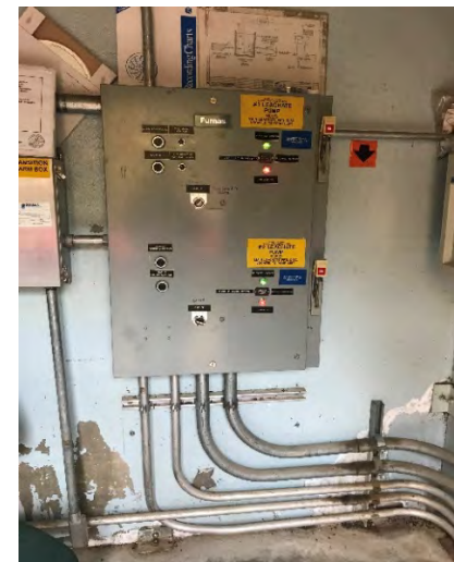
Leachate Pump Control Panel
