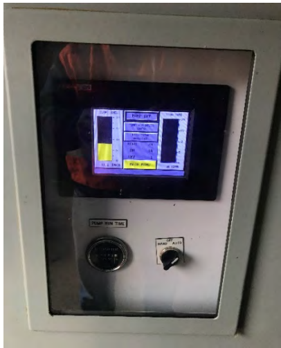
Leachate Pond Leak Detection Control Panel
