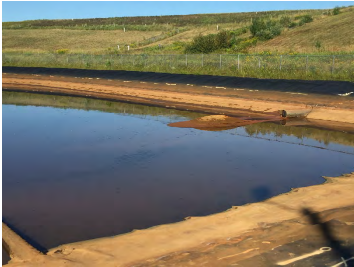
Sediment build-up at leachate pond inlet pipe
