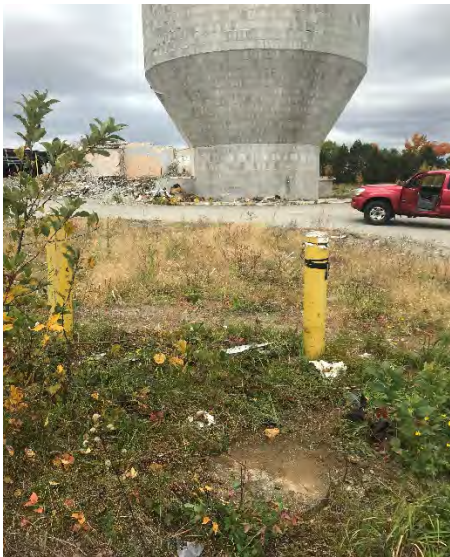
Leachate Pipeline Manhole at Former GNP Mill Site
