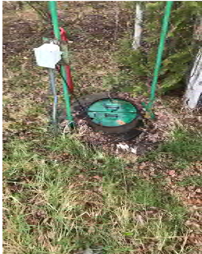
Leachate Pond Underdrain Pump Station
