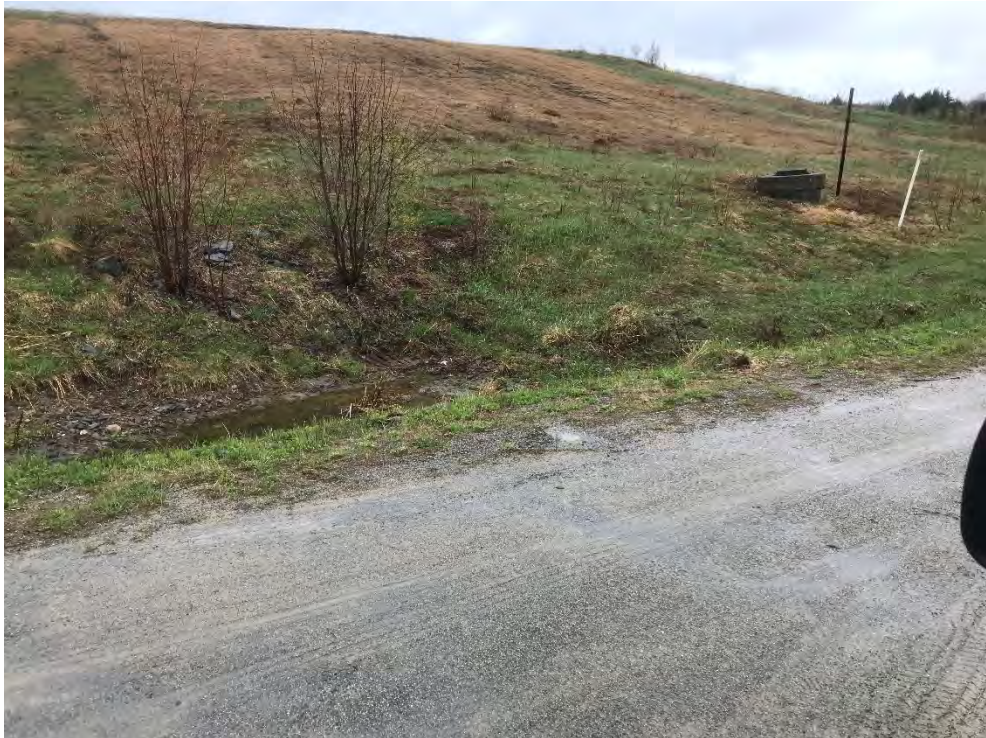
Dolby III Catch Basin (Item 10)
