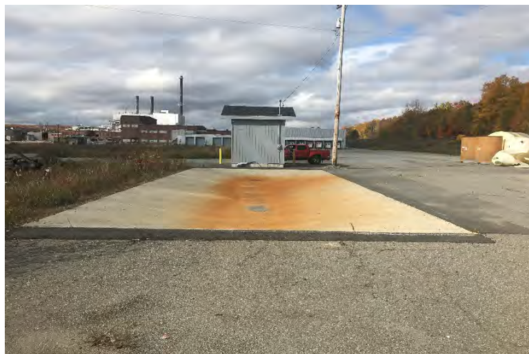
Emergency Leachate Unloading Area
