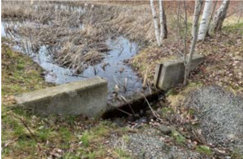
West Sediment Pond Outlet
