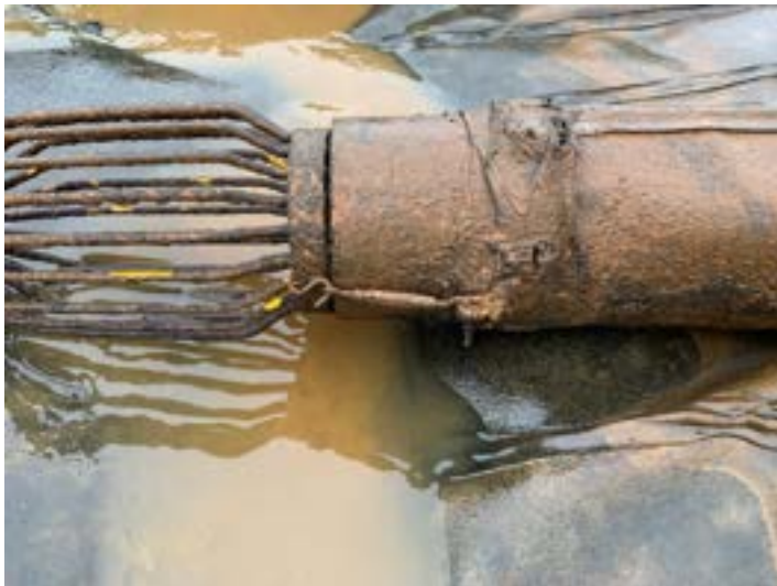
Condition of pumping outlet prior to repair
