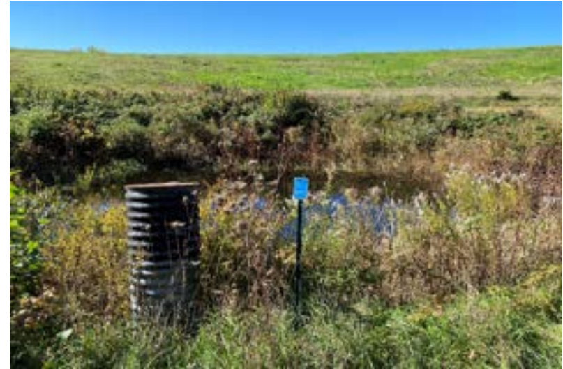
Dolby II Leachate Holding Pond
