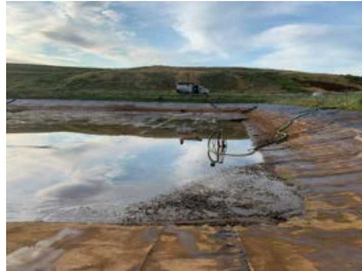
Sediment accumulation at Southwest corner
