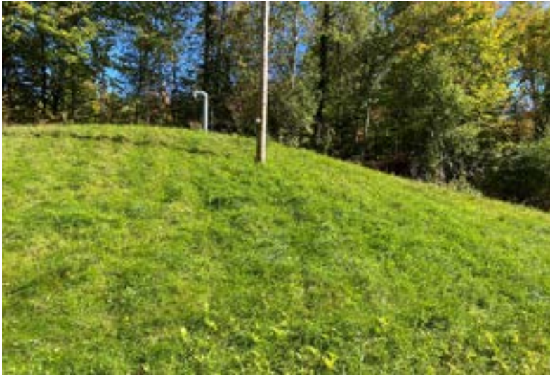
Leachate Transport Pipeline Transition Station
