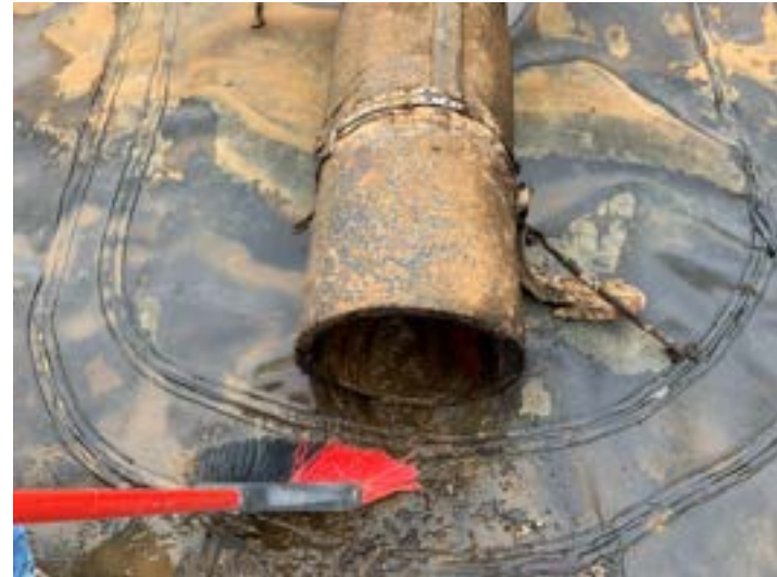
Existing caulking removed from outlet
