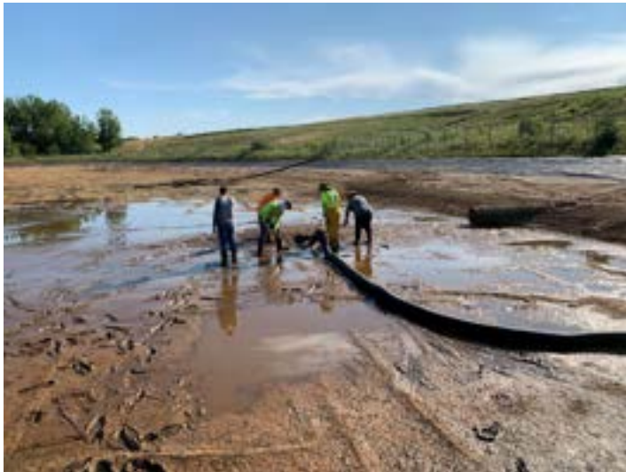
Cleaning inlet area
