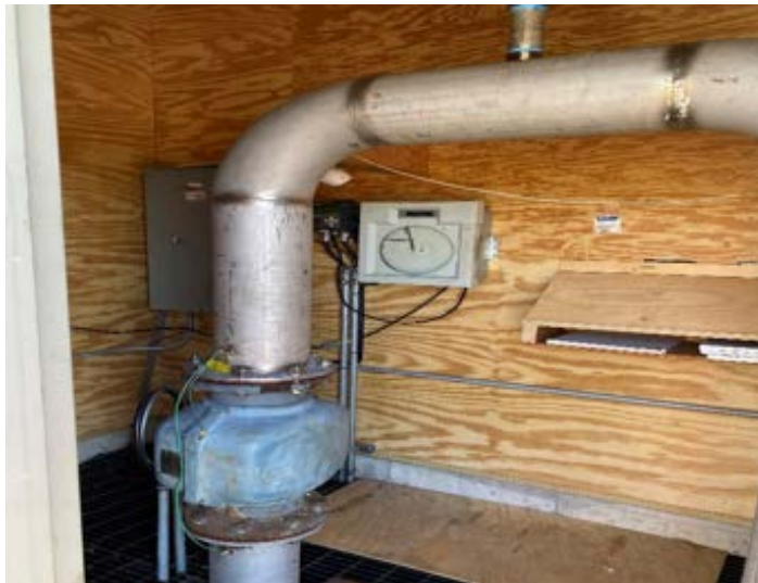
Leachate Transport Pipeline Flow Meter Building Interior
