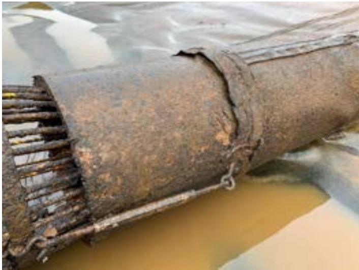
Condition of outlet prior to repair
