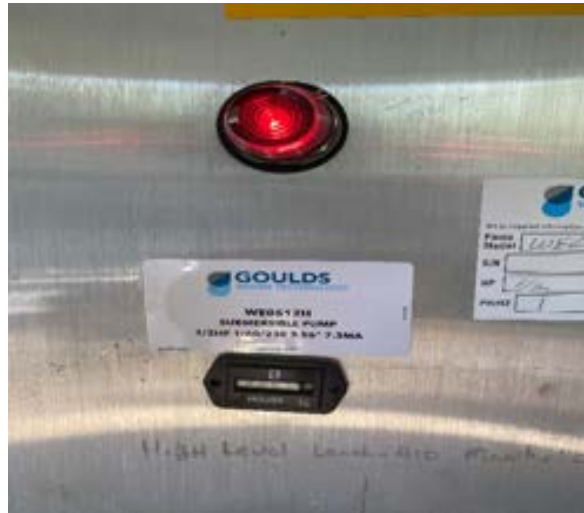
Leachate Pond Underdrain Run Time Meter
