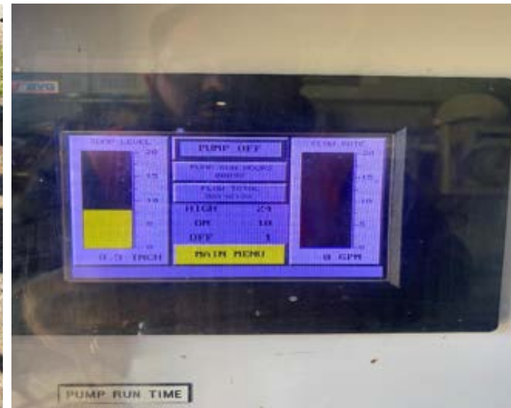
Leachate Pump Station Leak Detection Control Panel
