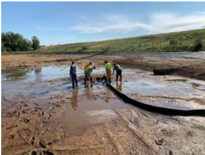
Cleaning inlet area
