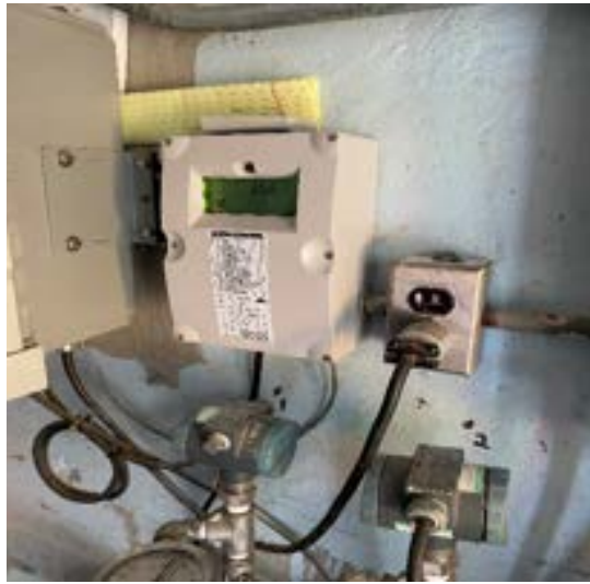
Leachate Pump Station Sonic Level Transmitter
