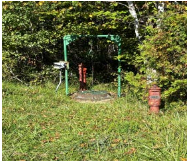
Leachate Pond Underdrain Pump Station
