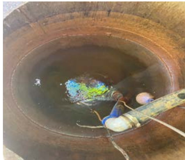
Leachate Pond Underdrain Pump
