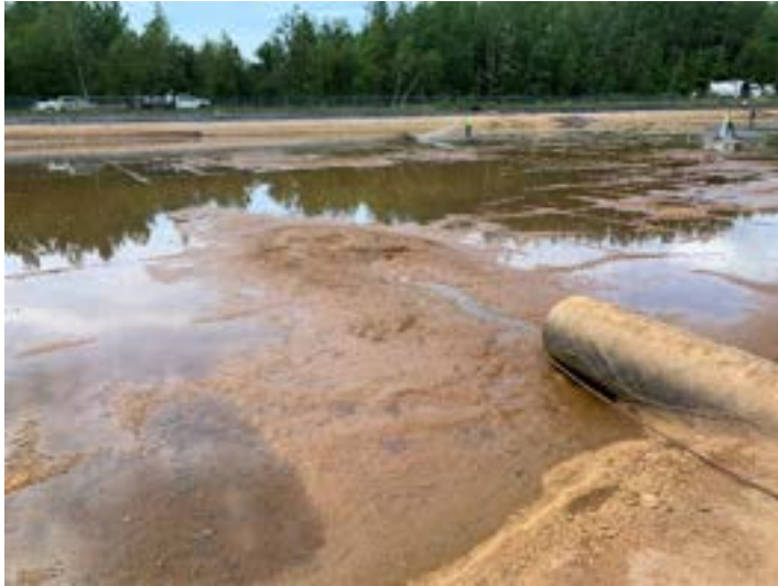
Sediment accumulation at leachate pond inlet pipe
