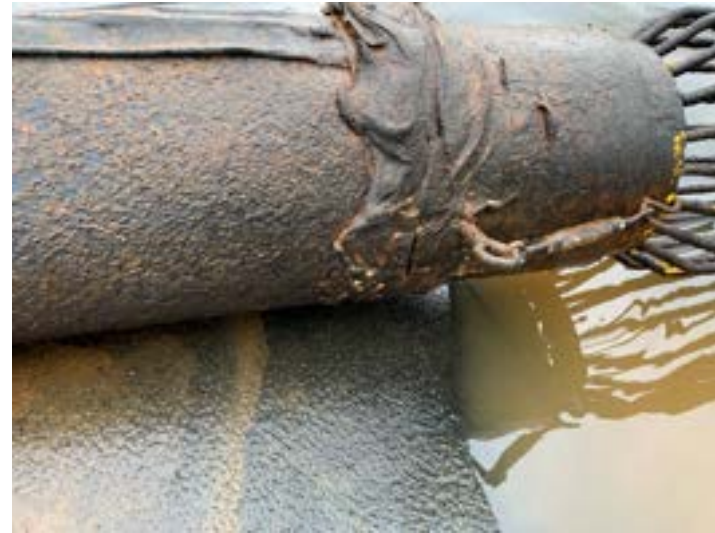
Condition of pumping outlet prior to repair
