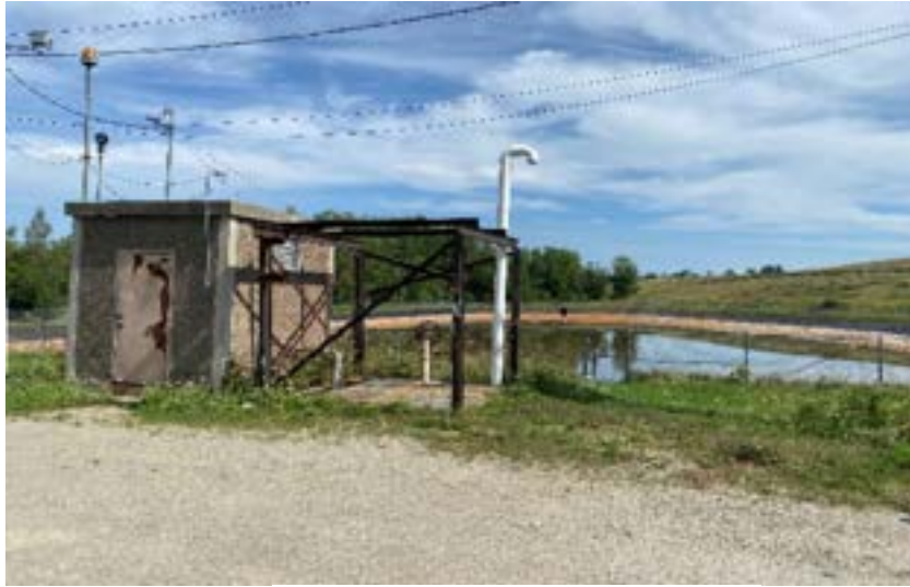
Leachate Pond and Pump Station
