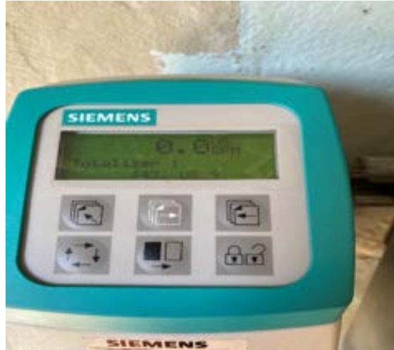
Leachate Pond Leak Detection Flow Transmitter
