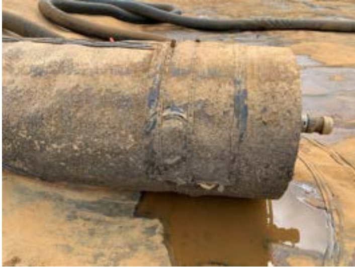
Condition of inlet prior to repair
