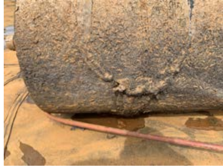
Condition of inlet prior to repair
