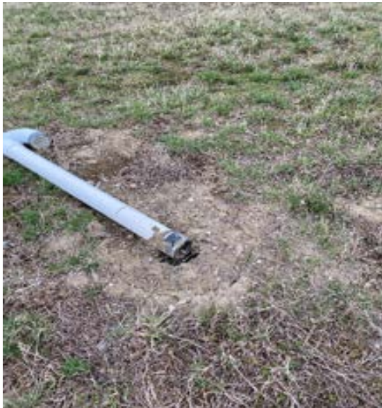
Dolby III Broken Gas Vent
