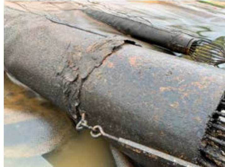
Condition of outlet prior to repair
