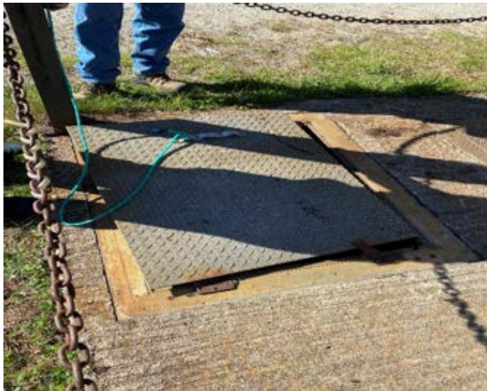
Leachate Pump Station Hatch Repair Needed
