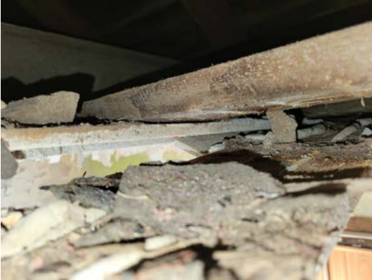
Roof shingle debris above Plaster Ceiling
