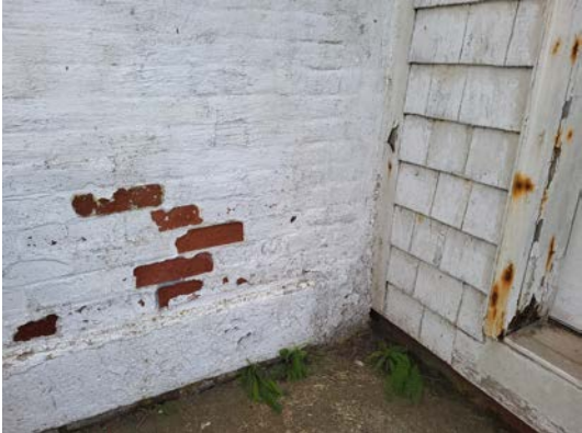
View of damaged coating on the exterior
