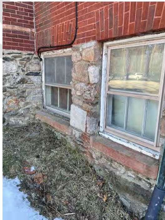
Image 83: Typical view of basement level wood windows. Notice deteriorated paint finish.
