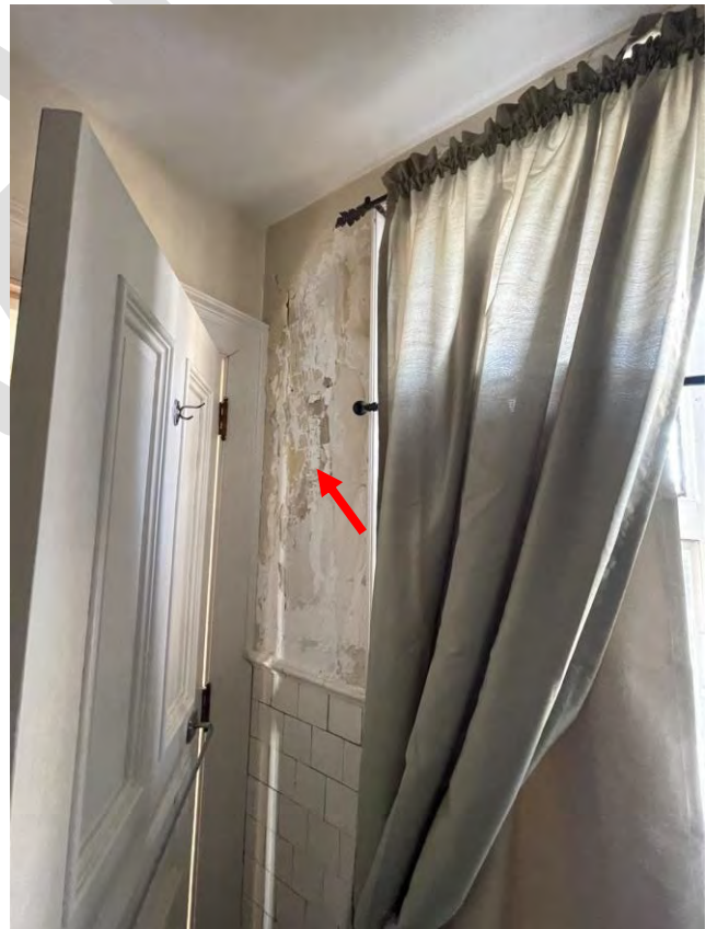
Image 7: View of water damage at first floor bathroom wall-southwest corner. Behind the bathroom door.
