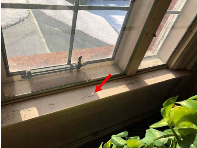
Image 12: View of painted interior windowsill with blistered and peeling paint.
