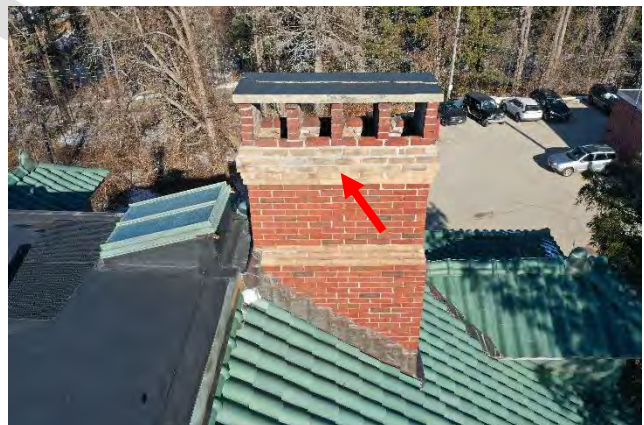
Image 19: View of chimney #3 that includes mortar deterioration in the yellow brick corbelling.
