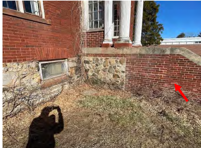
Image 39: View of opposite sidewall including deteriorated mortar joints, spalled brick, and poorly matched mortar repairs.
