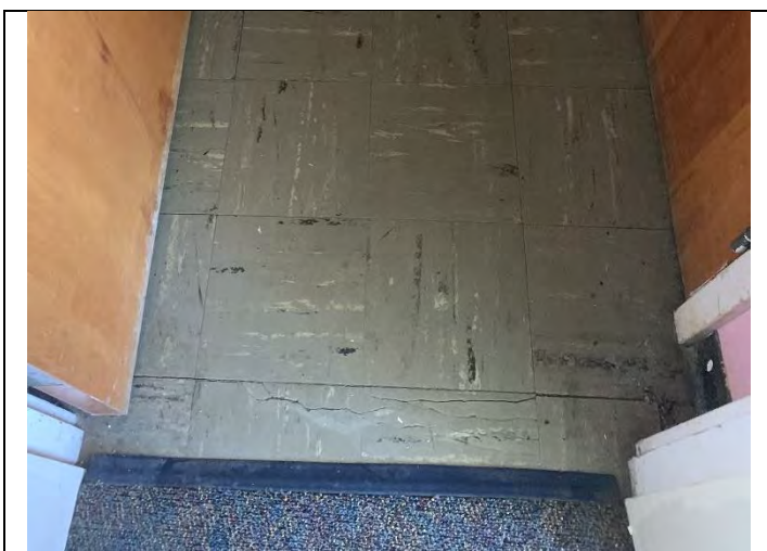
11. HG6 Grey 9" Floor tile with Mastic, in bathroom, kitchen and closets spaces throughout classrooms of Building G, to include under carpet and 12" Floor Tile
