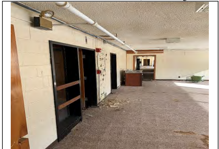
16. Building B 2 nd floor carpet – showing imprint of loose and damaged 9" ACM Vinyl Floor Tile underneath - throughout
