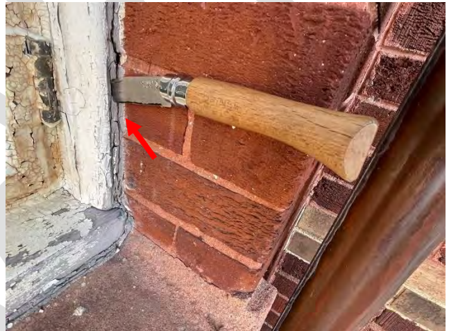
Image 87: View of typical deteriorated window perimeter sealant.
