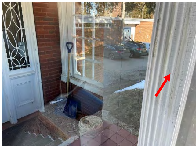
Image 47: View of interior of breezeway including cracked and peeling painted wood column.
