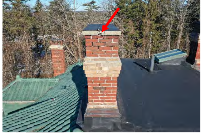
Image 15: View of chimney #1 that includes cracked cast stone cap, deteriorated and missing mortar, and poorly matched brick and mortar repairs.
