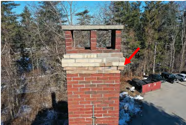
Image 16: View of chimney #2 that includes mortar deterioration, loose and displaced brick, and poorly matched brick and mortar repairs.
