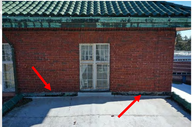
Image 69: View of the low sloped thermoplastic roofing system over the solarium roof with damaged copper throughwall flashing and deteriorated joint sealant.
