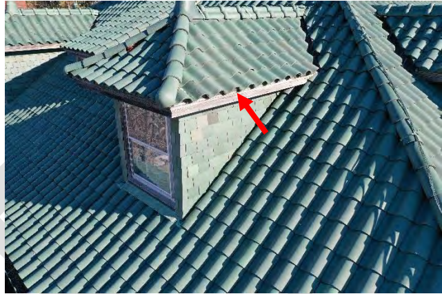
Image 55: View of typical dormer. Wood trim at eave and windows are bare wood.
