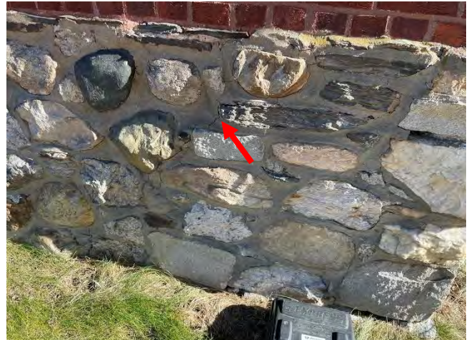
Image 29: Typical view of the existing stone foundation wall. Note the transverse crack in the mortar.
