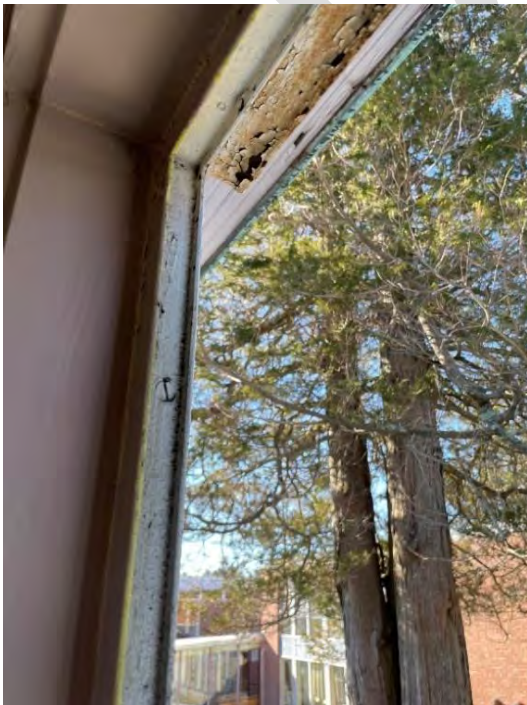
Image 82: Typical view peeling paint finish at steel window.
