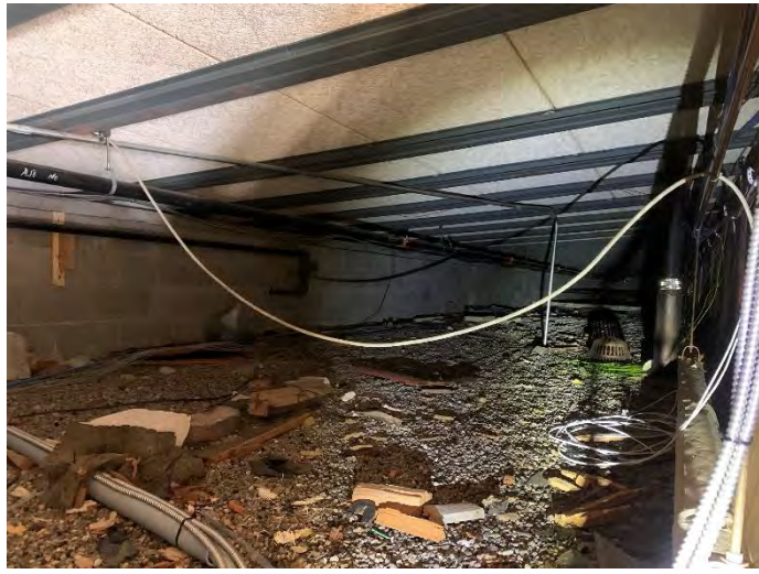
19. "Over-Roof" of Building G. Previous gravel roof left in place under new roof, and over hallway of Building G
