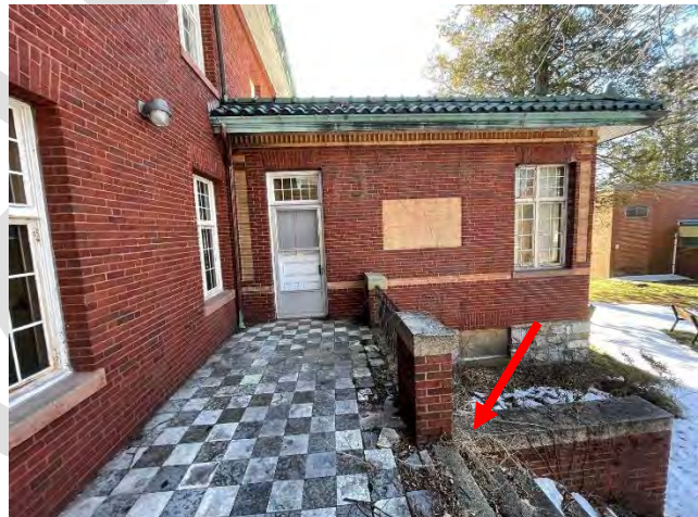
Image 49: Partial view of West entrance including environmental and atmospheric staining and plant growth.
