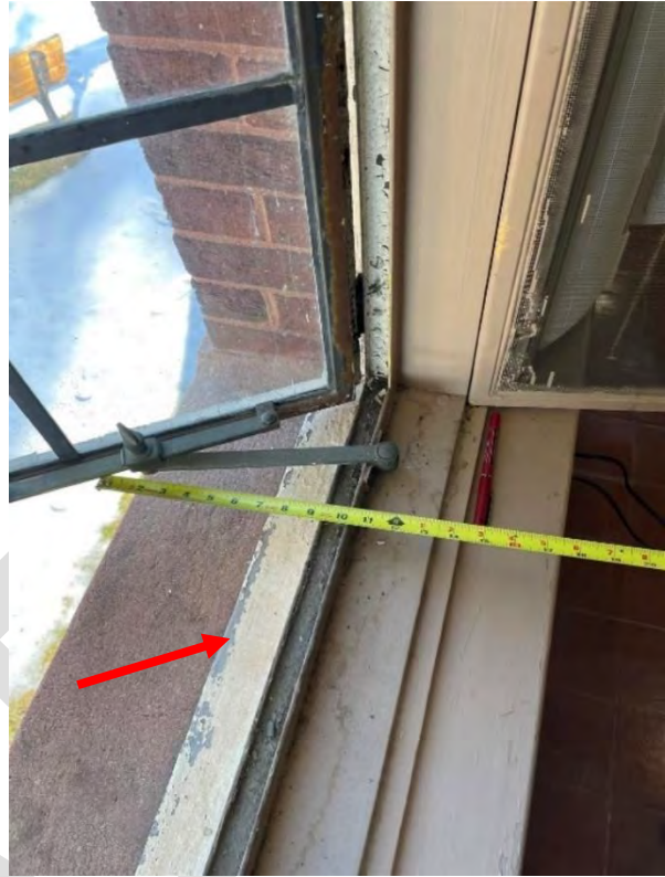
Image 81: Typical view peeling paint finish at steel window.
