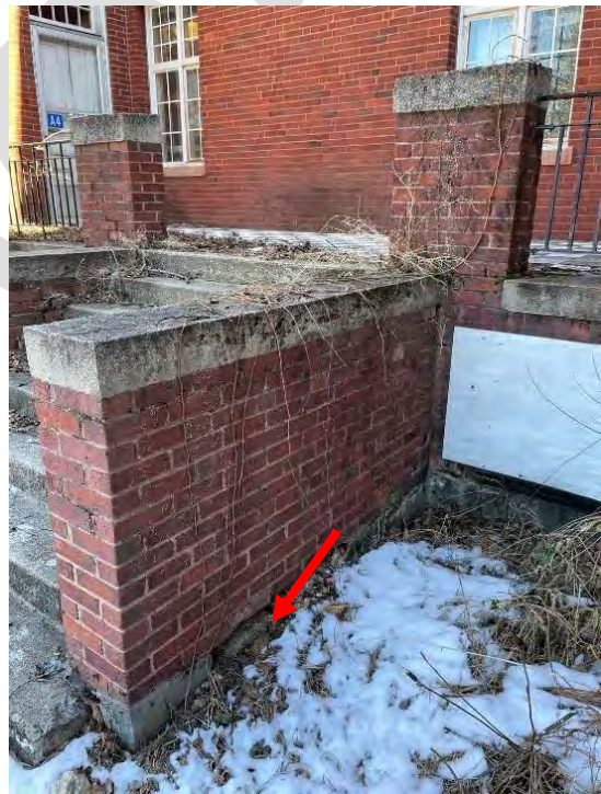
Image 53: View of eroded foundation, including deteriorated and missing brick.
