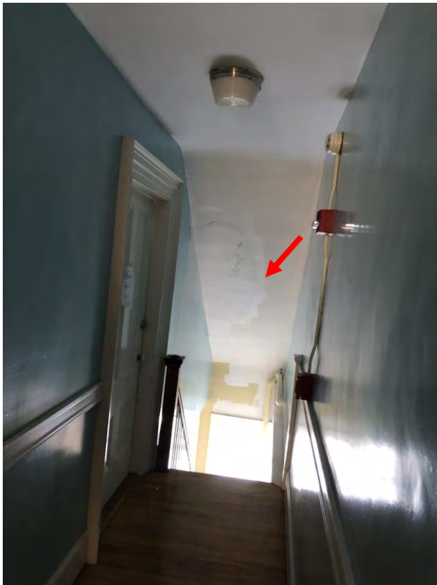
Image 10: View of water damaged ceiling in stairway
