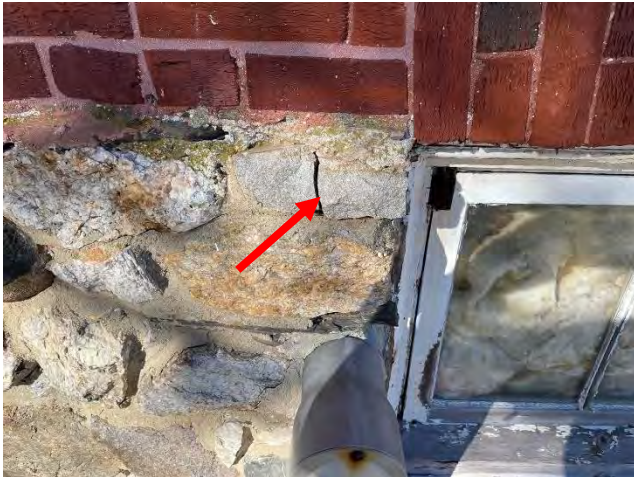
Image 28: View of cracked stone in foundation
