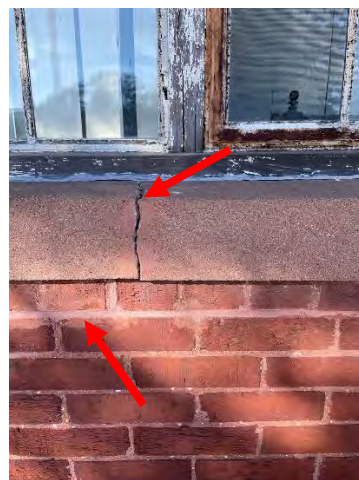
Image 27: View of crack cast stone sill and past mortar that were poorly matched to the existing.
