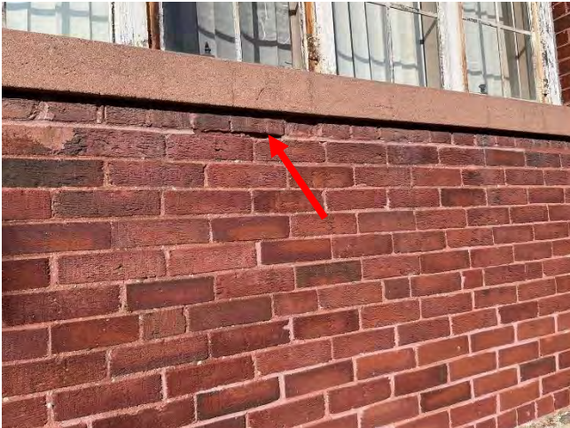
Image 22: Typical view of the existing red brick masonry and cast stone sill. Notice deteriorated mortar joint.
