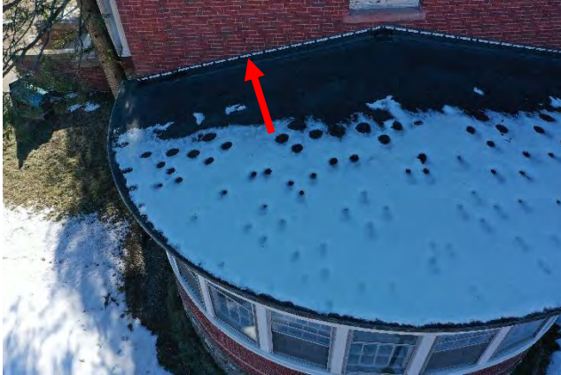
Image 66: View of elastomeric membrane roof over the Rotunda Room. Notice the absence of step flashing at the rising wall interface.
