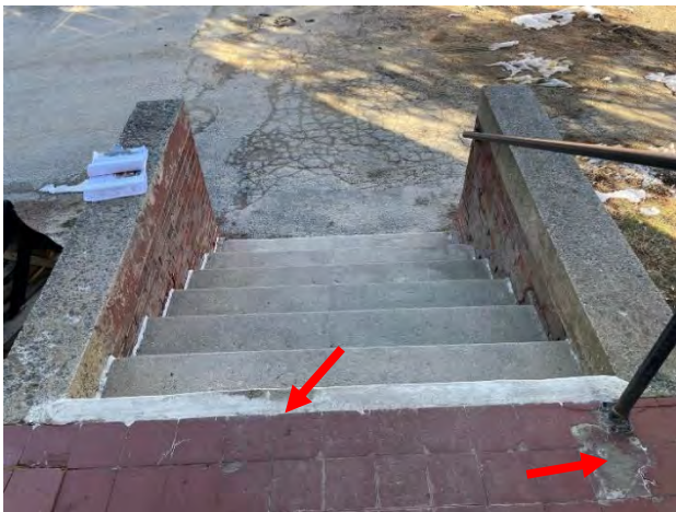
Image 44: View of poor patching at top step and railing base
