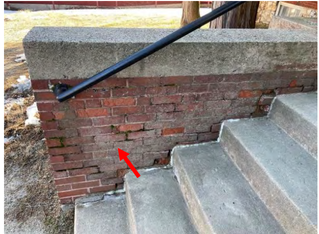
Image 43: View of deteriorated brick masonry stair sidewall including eroded mortar joints, spalled and displaced brick, and deteriorated joint sealant.
