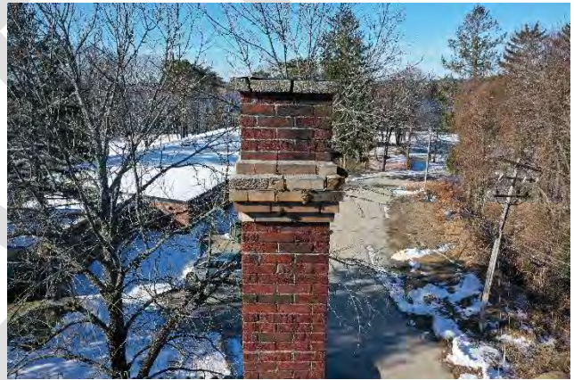
Image 17: Side view of chimney #2 that includes deteriorated mortar joints, loose and displaced brick at the yellow brick banding and cracked cap.
