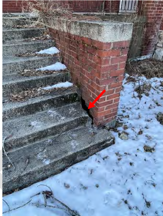
Image 51: View of deterioration of the concrete foundation, deteriorated and missing brick and mortar joints, missing joint sealant at steps, as well as dormant vine growth.
