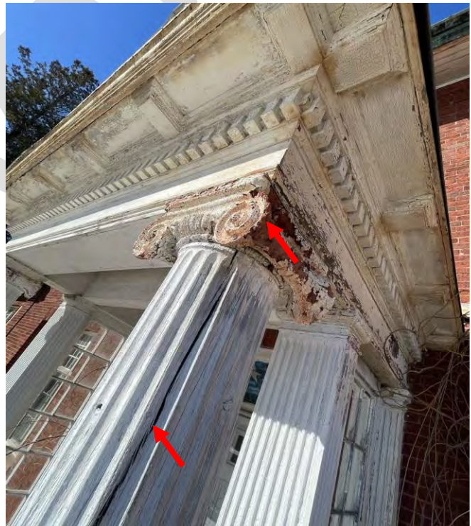
Image 33: View of the Ionic column volute and abacus that are severely deteriorated. Also notice the painted wood column is split.
