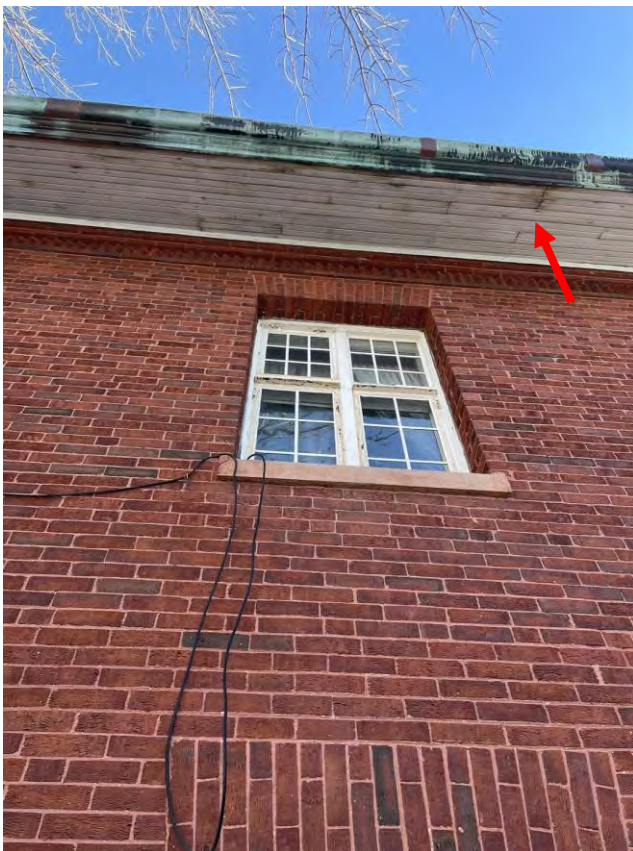
Image 72: Typical view of the existing wood bead board soffit paneling. Notice dirt and moisture staining.
