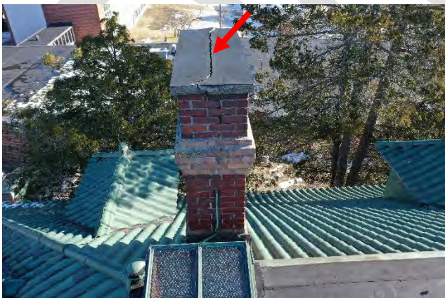
Image 18: View of chimney #3 that includes cracked cast stone cap, severe mortar deterioration and poorly matched brick and mortar repairs.
