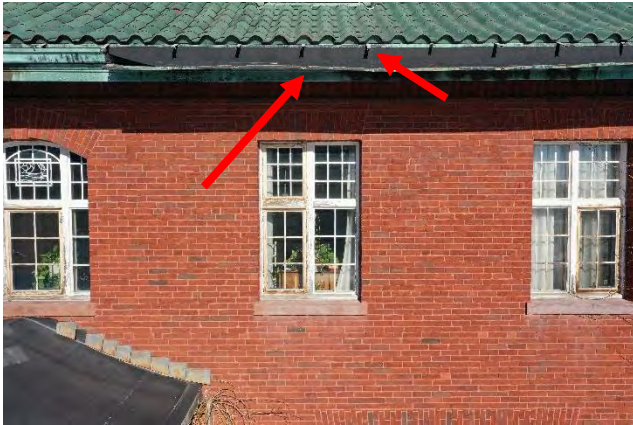
Image 70: View of damaged and broken gutter, and gutter brackets.
