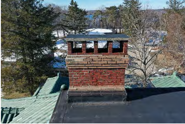
Image 14: View of chimney #1 that includes mortar deterioration, loose and displaced brick, poorly matched brick and mortar repairs.
