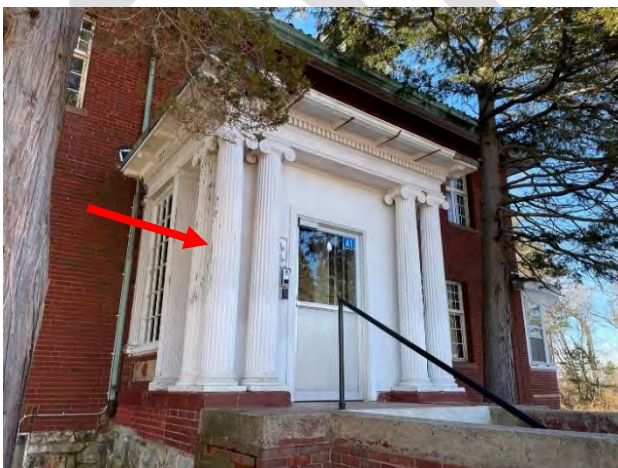
Image 40: Overall view of East entryway including enclosed breezeway with aluminum entrance door. Also notice peeling paint on the wood columns.
