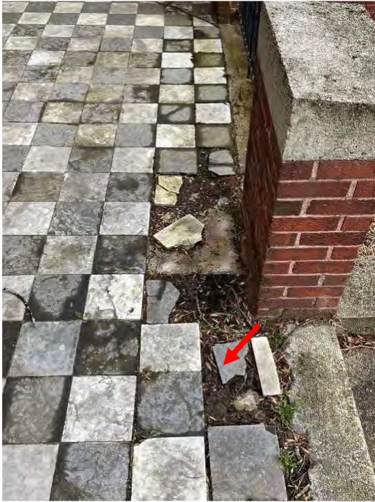
Image 50: View of marble tile pavers that are delaminated, broken, and displaced unevenly.
