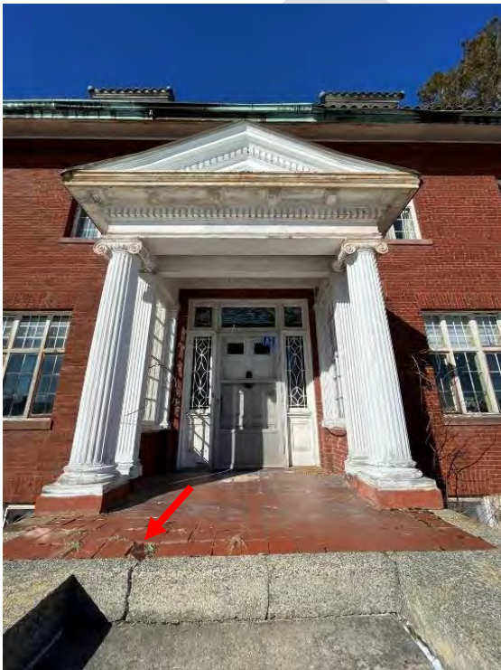
Image 32: Overall view of the south entrance with broken, displaced, and uneven clay tile pavers and cracked concrete steps.
