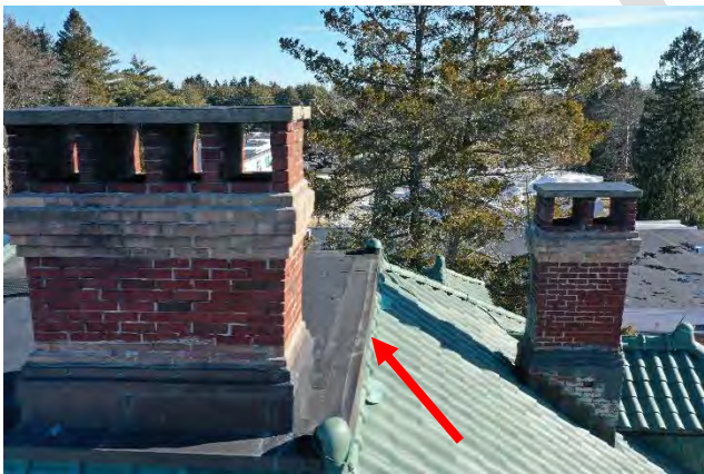
Image 64: View of the perimeter flashing, and edge metal fascia overlap the terra cotta tile ridge caps.
