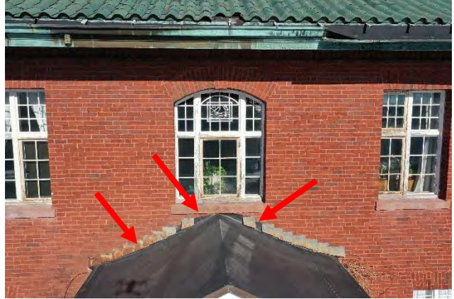
Image 67: View of the south entrance including missing and rust corroded step counterflashing. Note that the roof to wall transition where the flashing is missing is open to the weather.
