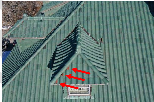
Image 57: Another typical view of the Terra Cotta Spanish tile roofing including hip and ridge caps and finials. Notice the broken terra cotta tiles.
