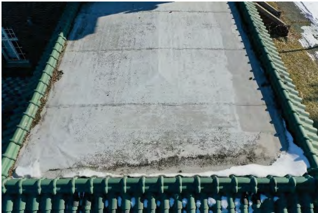
Image 68: View of the low sloped thermoplastic roofing system over the solarium roof and surrounded by terra cotta Spanish tile mansard.
