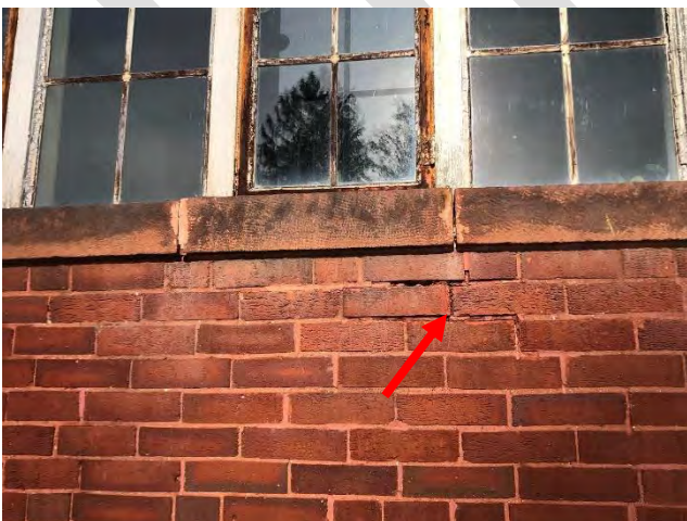
Image 26: View of eroded brick and cast stone sill mortar joints.
