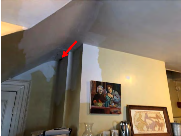
Image 8: View of water damaged plaster patching
