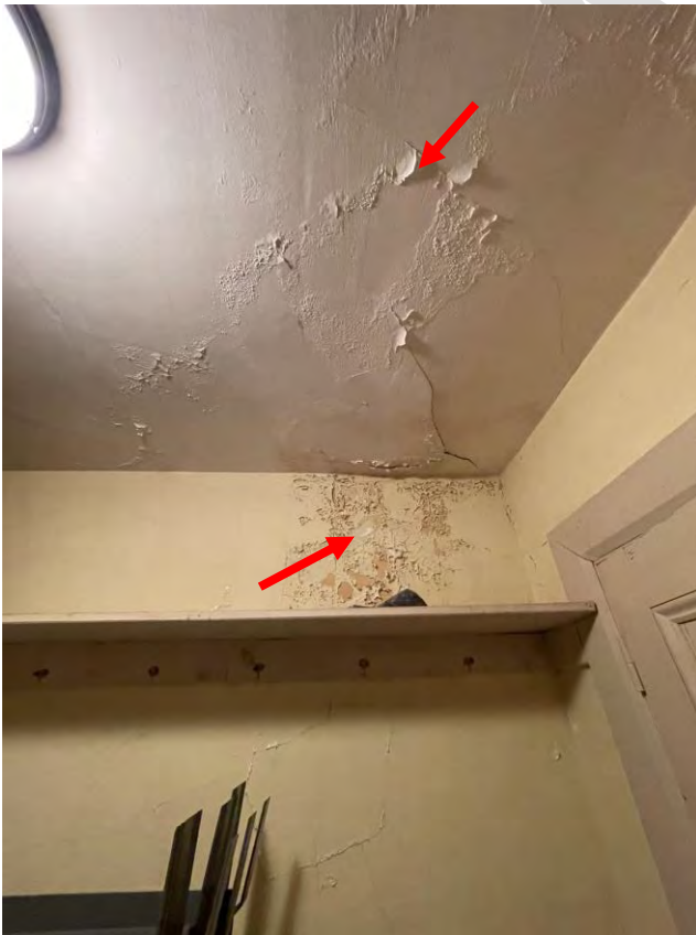
Image 6: View of water damage at second floor closet ceiling and wall.
