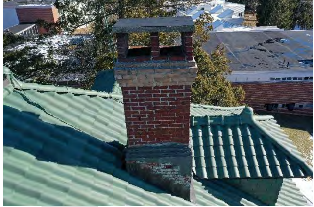
Image 21: View of chimney #4 that appears to have been rebuilt but with poorly matching and applied mortar. Also, notice bituminous mastic repairs.
