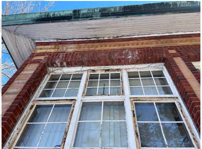
Image 79: Another view of steel framed windows and in wood frames notice deteriorated paint and with rust corrosion.
