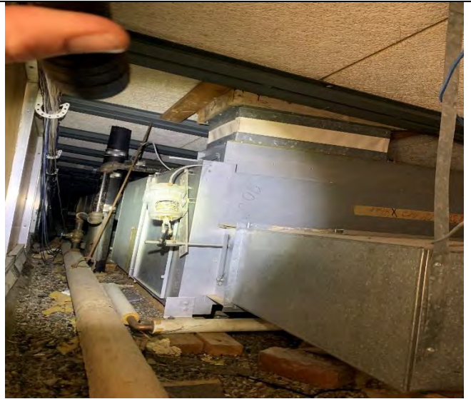
20. "Over-Roof" Space contains some Mudded Fittings in Fiberglass Pipe Insulation runs - HG26 ACM
