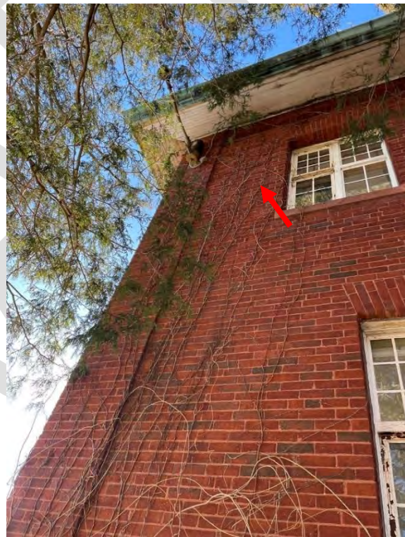
Image 31: View of vines growing up the brick wall near the southeast corner
