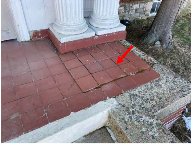
Image 42: View of broken, displaced, and uneven tile pavers.
