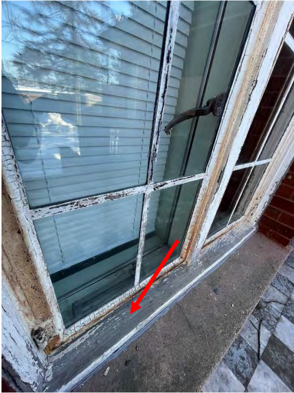
Image 80: Typical view of deteriorated paint finish and exposed bare wood.
