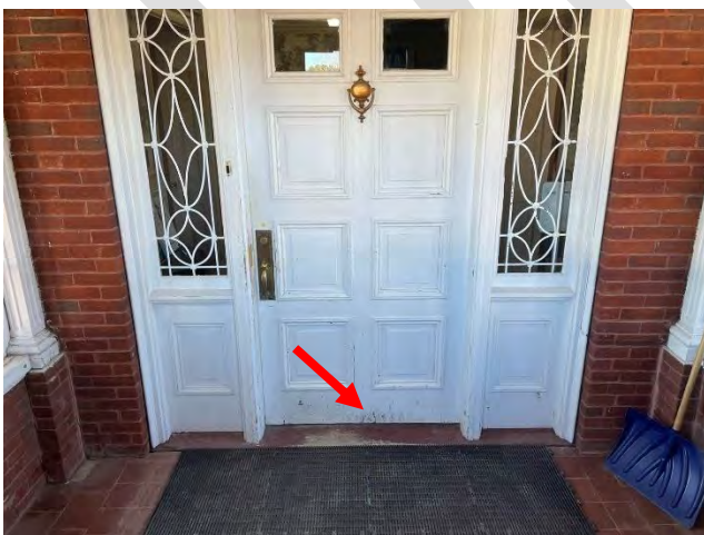
Image 46: View of exterior door within the enclosed breezeway including peeling paint.
