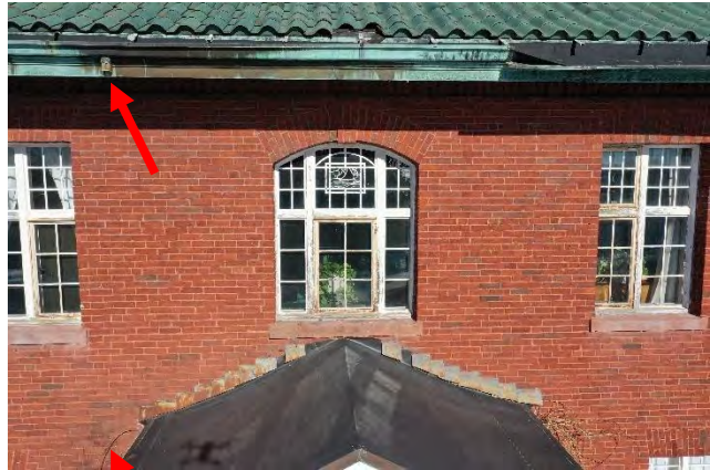
Image 71: View of missing downspout leader.
