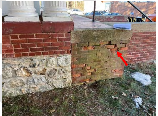
Image 45: View of side of porch including mortar deterioration, spalled and displaced brick, and algae growth.
