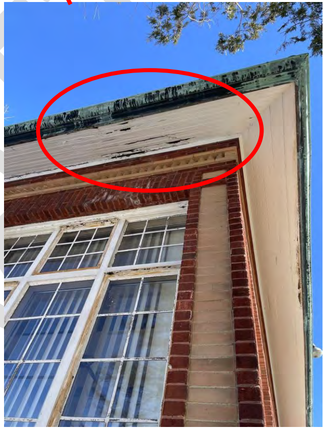
Image 73: View of the existing wood bead board soffit paneling. Notice that wood appears to be rotted and decayed.
