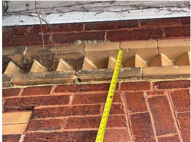
Image 23: View of decorative yellow brick banding with deteriorated mortar joints.
