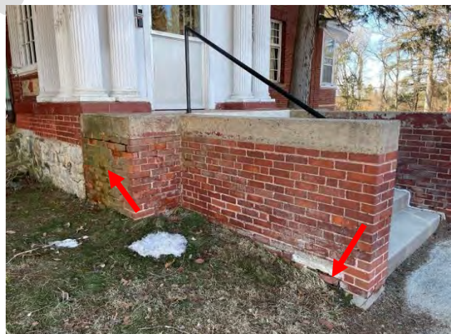
Image 41: View of deteriorated brick masonry and organic algae staining on the brick masonry stair sidewalls.
