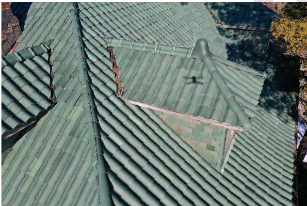
Image 56: Typical view of the Terra Cotta Spanish tile roofing including hip and ridge caps and finial, and flat shingle tile on the sides of the dormer.
