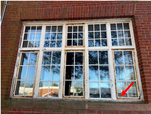
Image 78: View of steel framed windows and in wood frames notice deteriorated paint and with rust corrosion.
