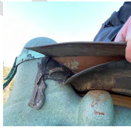
Image 65: View of edge metal fascia lifted and exposing wood blocking and underlying roof.
