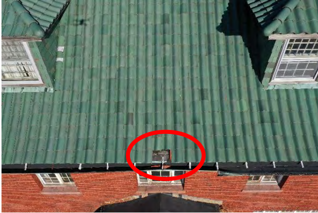
Image 58: View of broken and missing roofing tiles at the gutter roof edge of the south elevation.
