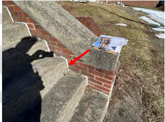
Image 37: View of deteriorated joint sealant between stair steps and the brick masonry.
