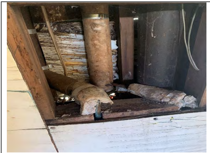
7. HG25 ACM Mudded Fitting, Building B where removal occurred at bathroom or kitchen spaces
