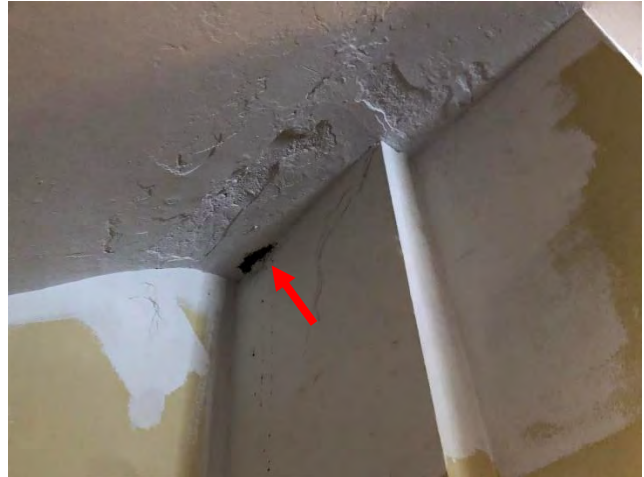
Image 9: View of damaged plaster ceiling
