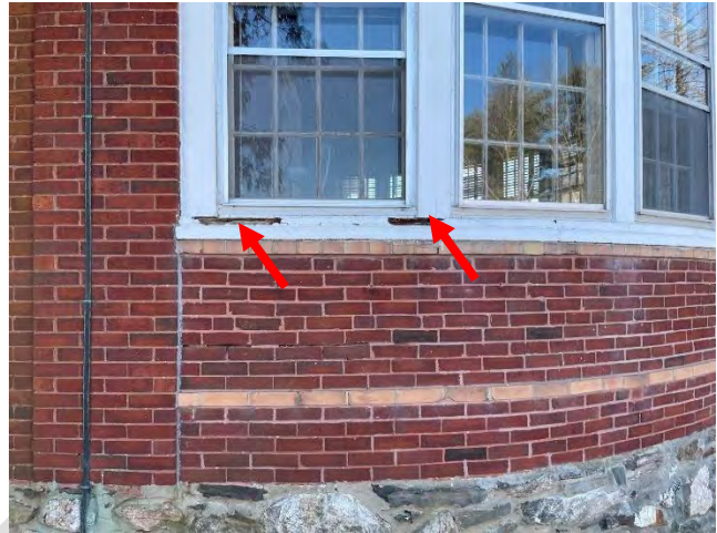
Image 85: View of rotted and decayed wood sills.
