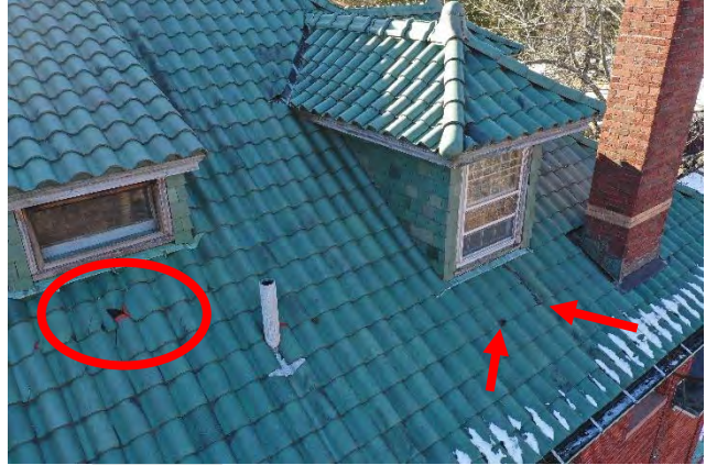
Image 59: View broken roofing tiles and roof mastic repairs.
