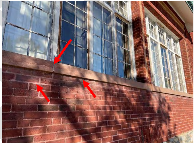
Image 25: View of cracked cast stone sills, spalled brick and poor mortar match at repair locations.
