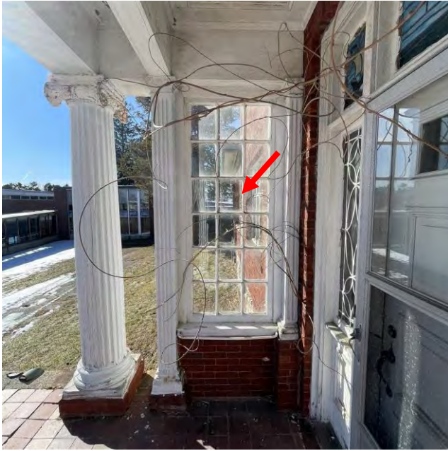
Image 34: View of the painted wood entry sidelights. Sidelights are deteriorated and missing glazing putty.
