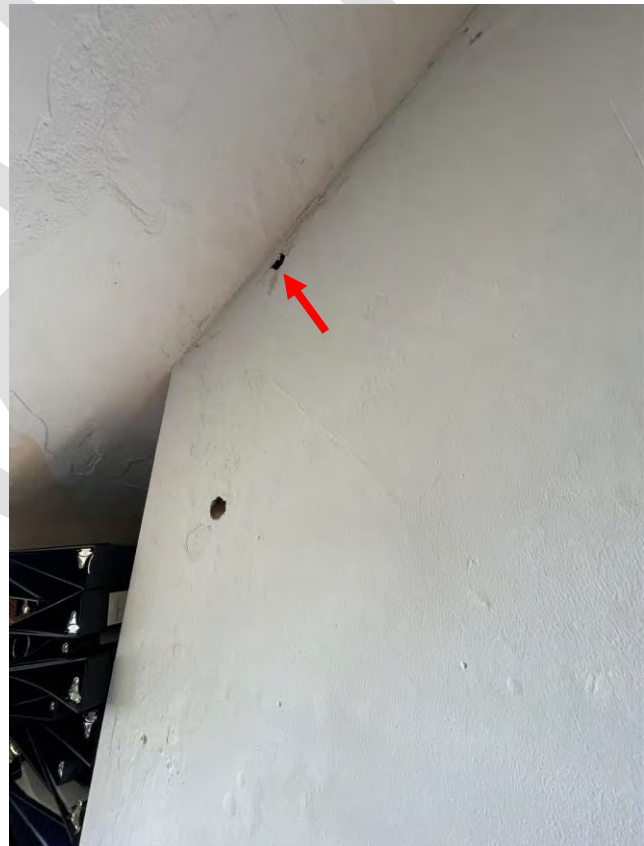
Image 11: View of water damaged plaster.
