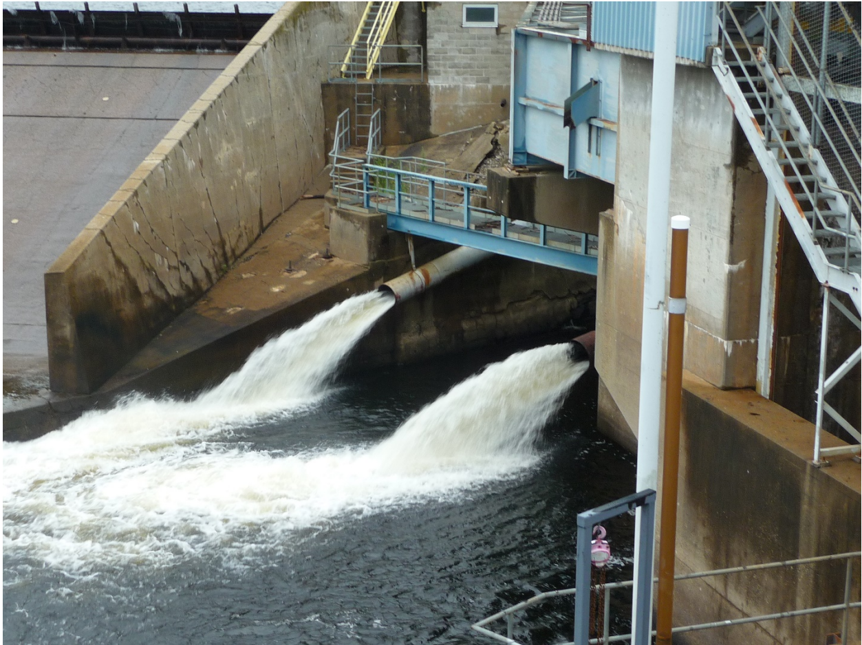
Figure 2.1.3.2-2: Downstream Fish Passage Facility Transport Pipes
