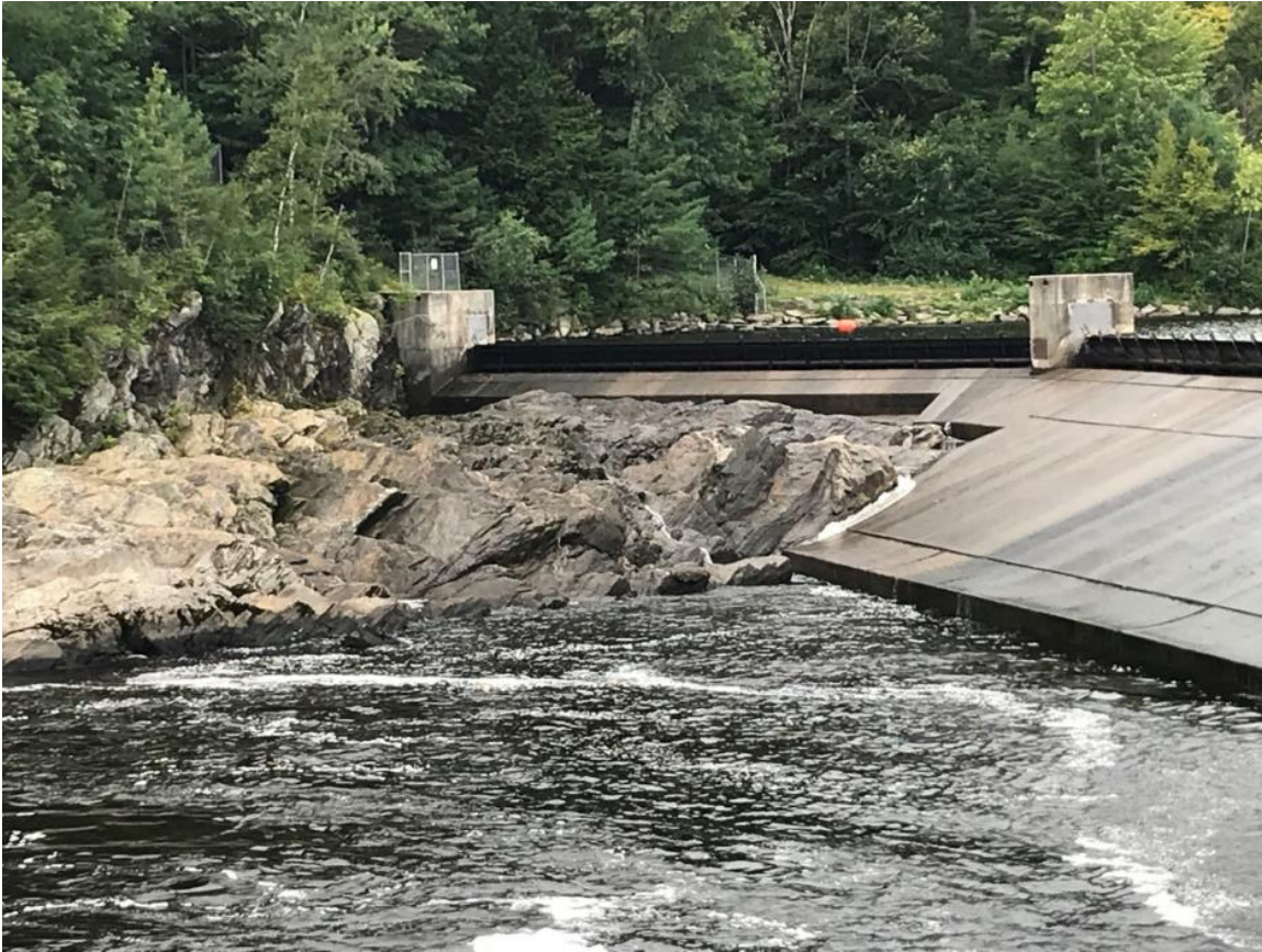
Figure 4.6.1.3.2-3: Exposed Bedrock Area below Bascule Gate No. 5 as Viewed from River Left
