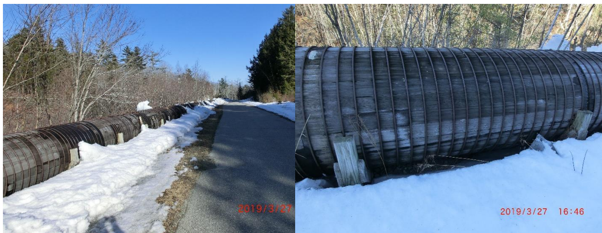
Photo 2-6 Wood Stave Penstock
