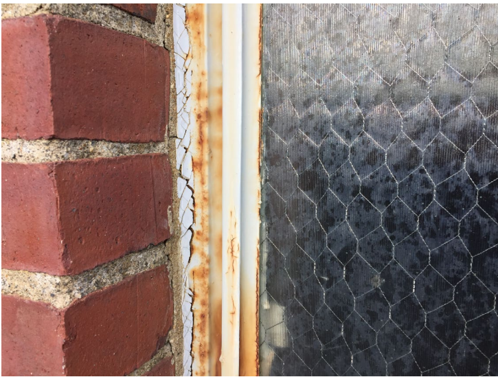
Asbestos-containing caulk on Screen House 1 exterior (Sample set C-11)
