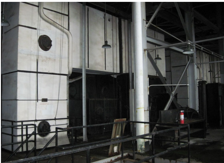
Boiler units and ductwork with ACM thermal jacketing/lagging
