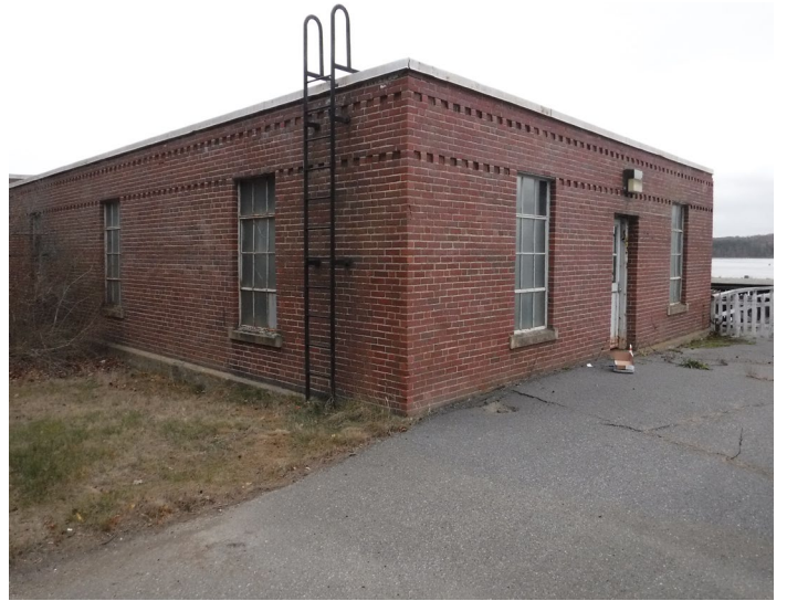
View of Screen House 1, including windows with ACM glazing (Sample set SH-04)
