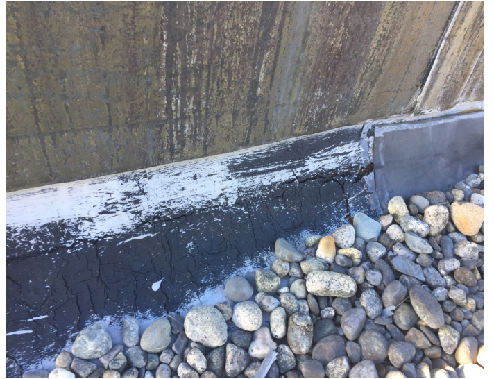
ACM roof flashing materials on rear (west) elevated roof section, and Units 3&4 upper areas (Samples R-16 - R-19)
