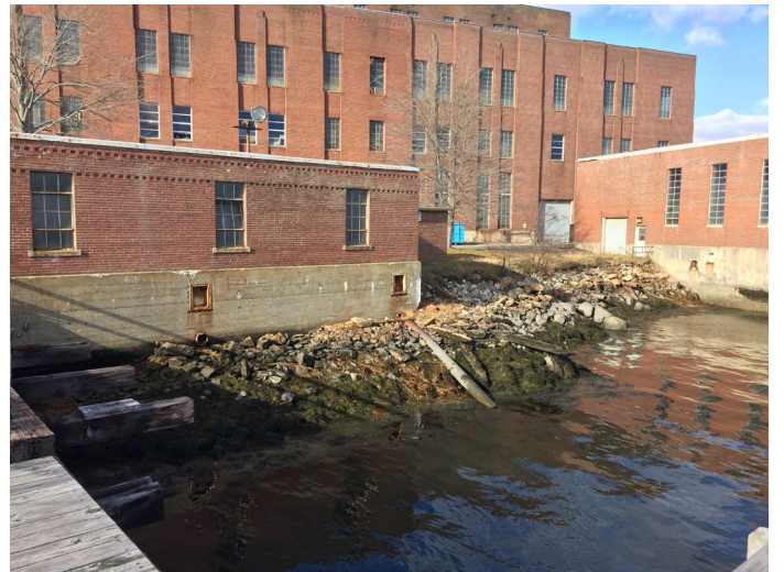
View of Screen House 1 (L) and Screen House 2 (R). Screen House 2 also has ACM window glazing (Sample set SH-01)
