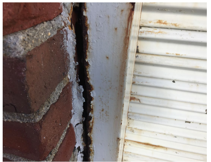
Closer view of asbestos-containing caulk on Screen House 2 exterior doors
