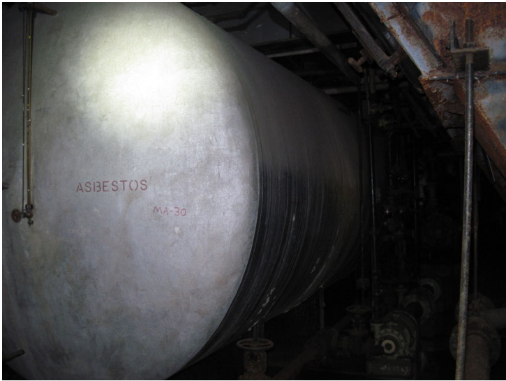
One of several large-diameter tanks with ACM jacketing observed throughout Powerhouse Building
