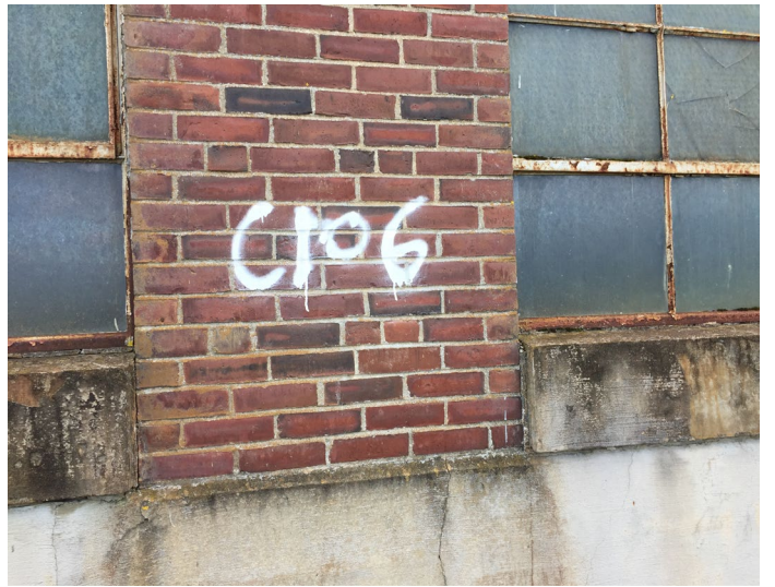
Asbestos caulk on Units 3&4 windows, north elevation (Sample set C-06)
