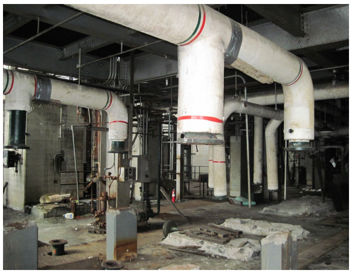
Large-diameter water and steam piping observed throughout Powerhouse Building interior
