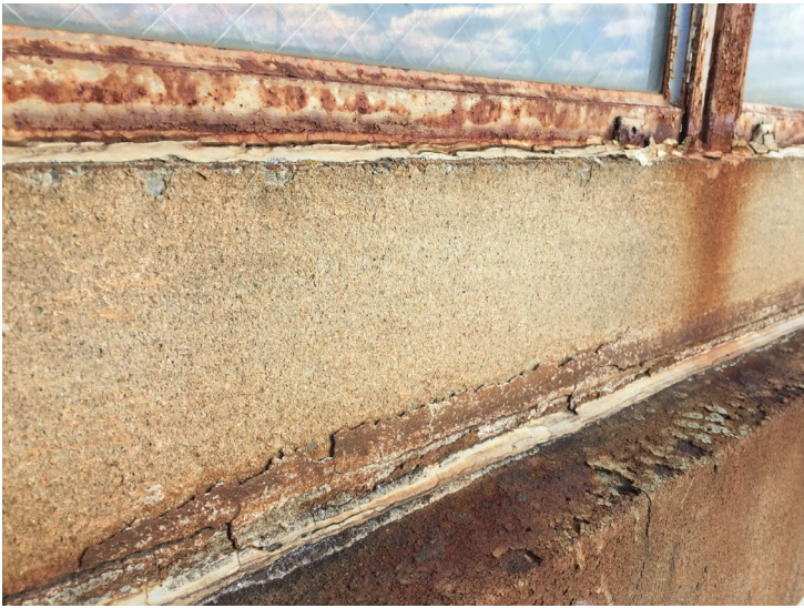
Closer view of ACM caulk on Unit 5 windows
