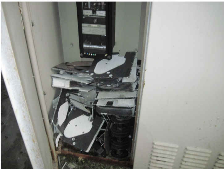
Closer view of asbestos-cement pieces within electrical panels. Black = sample set 16, gray = PACM
