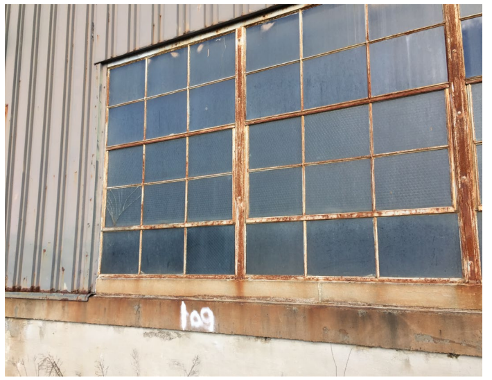
Asbestos caulk on Unit 5 windows, south elevation (Sample set C-09)
