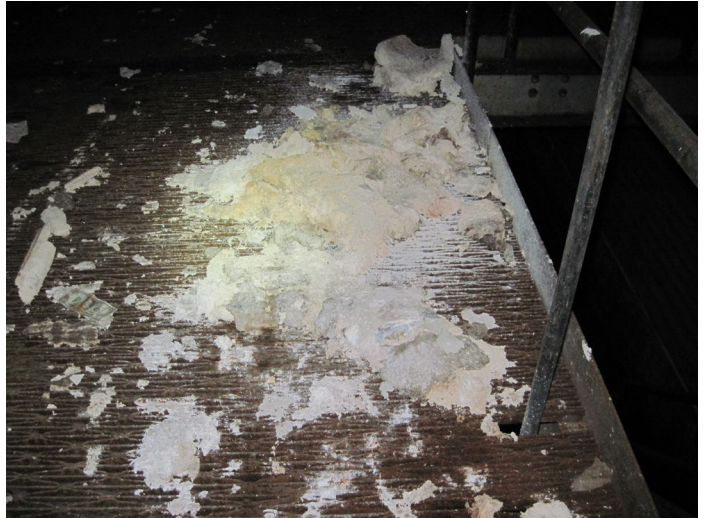
Asbestos-containing debris noted in several locations throughout Powerhouse Building interior
