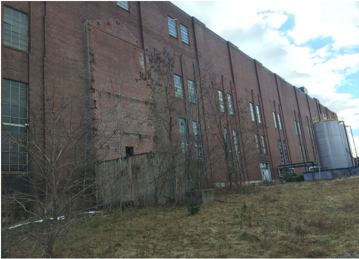
View of the rear (west) elevation of the Powerhouse Building. View is to the southeast.
