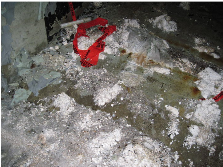
ACM debris on floor due to overhead water damage to pipe and unit insulation
