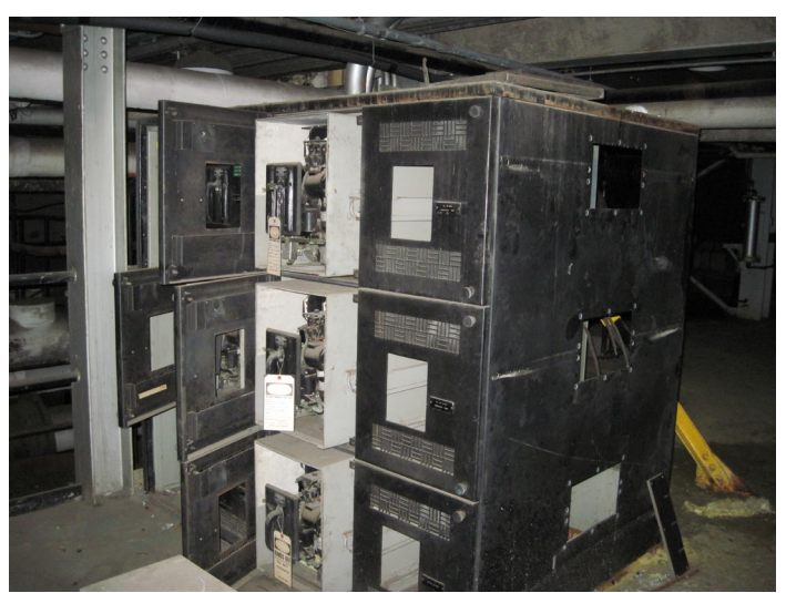
One of several electrical cabinets containing asbestos-cement paneling and other components
