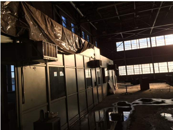
Wall-mounted air conditioners observed in Powerhouse Building interior, to be managed as universal wastes.
