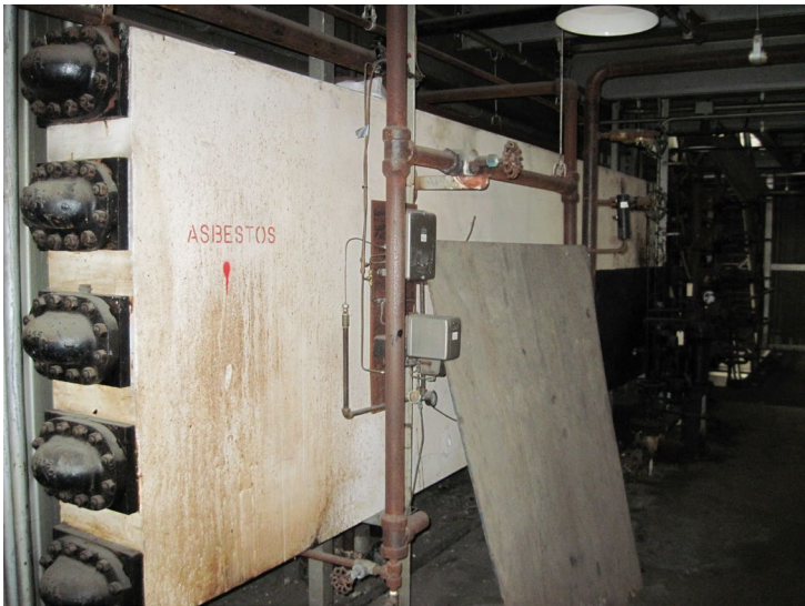
Oil heater unit appears to be only remaining ACM-insulated process equipment in Unit #5 area.
