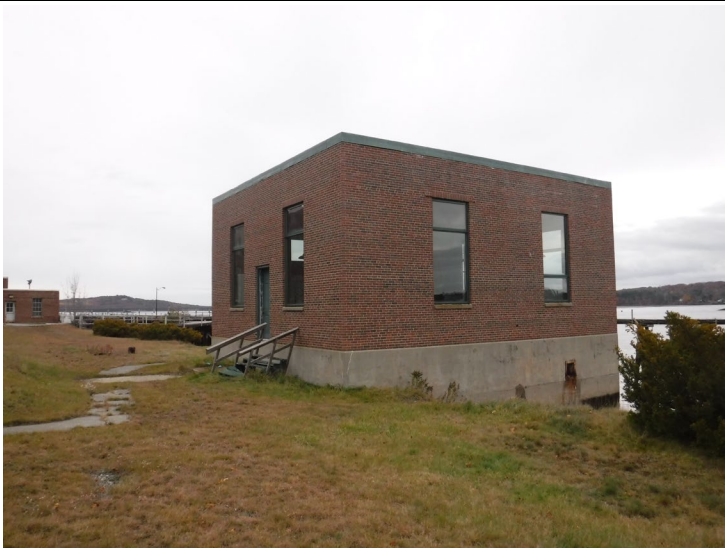
View of Screen House 3. Only ACM identified is small quantity of caulk on concrete foundation (Sample set C-10)
