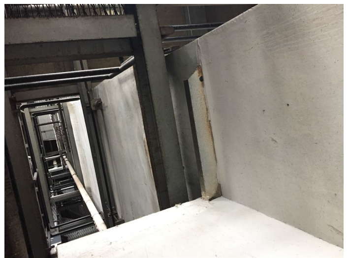
Vertical view of ACM jacketing on multi-story boiler process equipment
