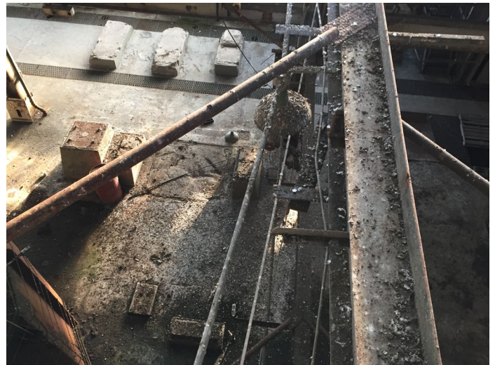
View of pigeon droppings, widespread throughout Unit 5 areas, ground floor.
