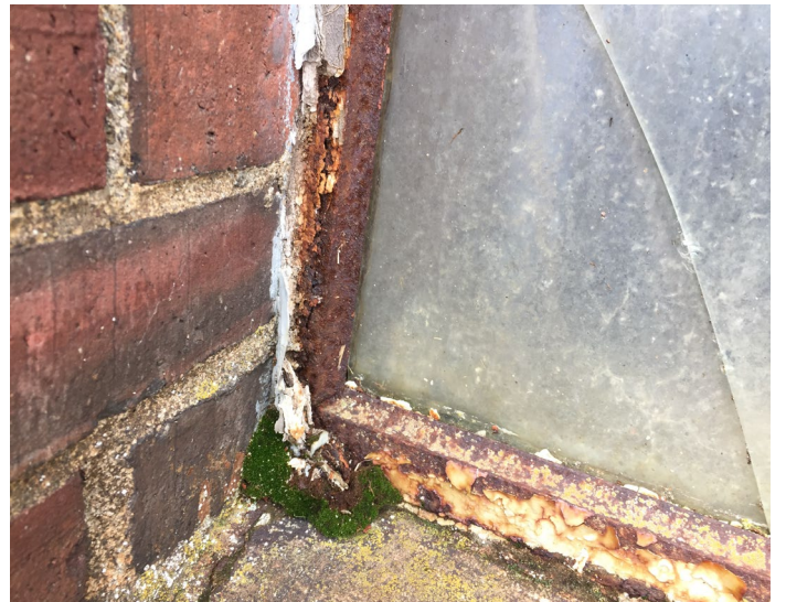
Closer view of ACM caulk on Units 1&2 windows
