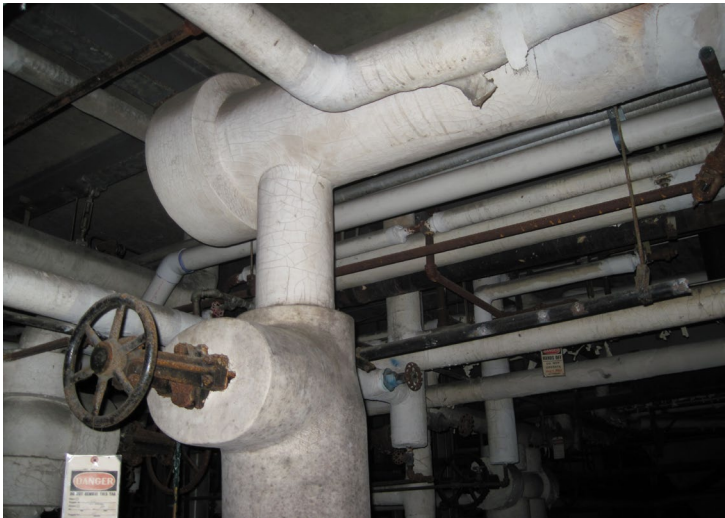
Small-diameter ( \leq 18'' D) piping observed throughout Powerhouse Building interior
