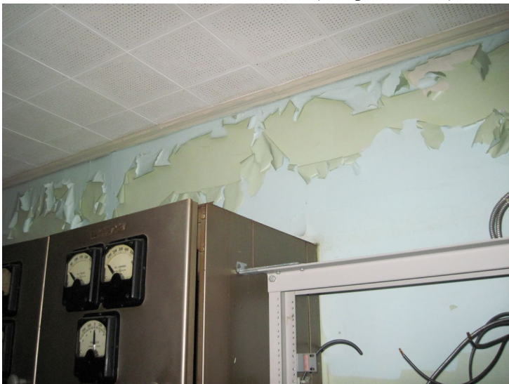
PCB-containing paint on interior plaster walls within CMP control room, 3 rd floor of Powerhouse Building (Sample P-07)
