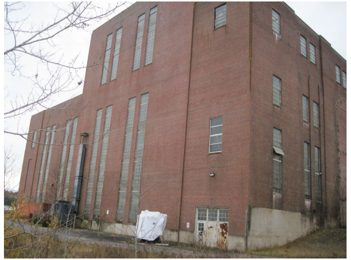
View of the north elevation of Powerhouse Building. View is to the south.
