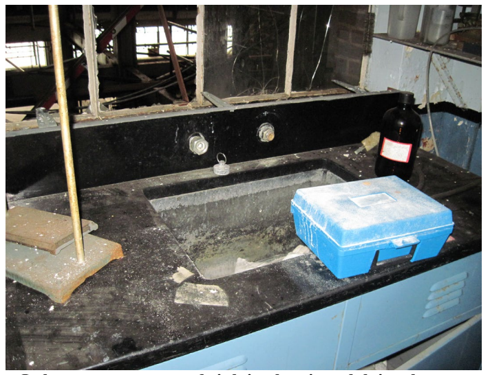
Lab countertop around sink in chemistry lab is asbestos-cement (Sample set 11)
