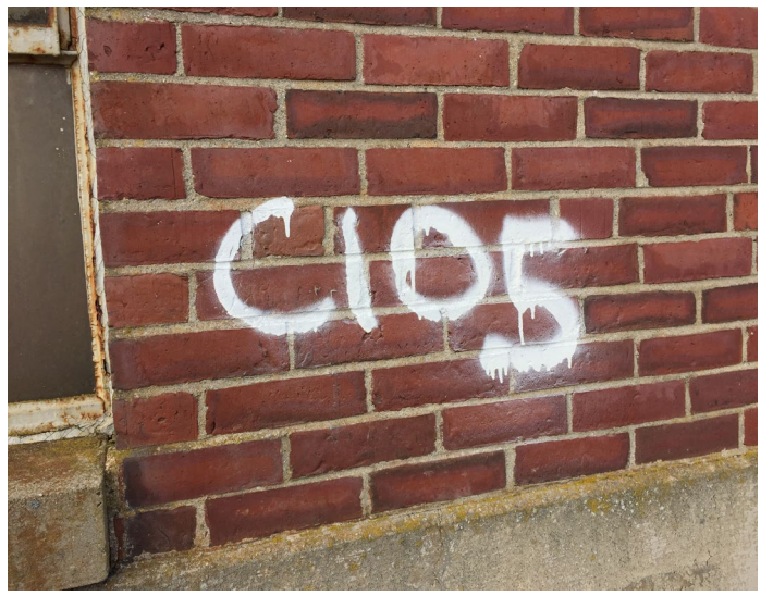
Asbestos caulk on Units 3&4 windows, east elevation (Sample set C-05)
