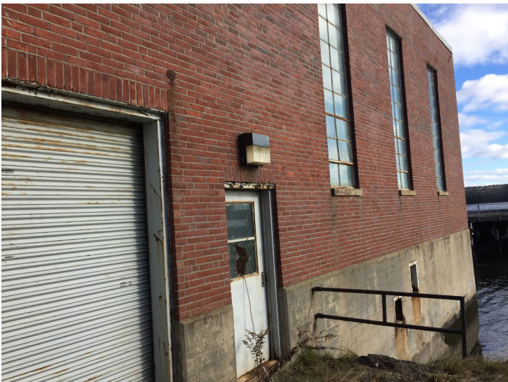
View of overhead and entry doors on Screen House 2, both with ACM perimeter caulk (Sample set C-12)
