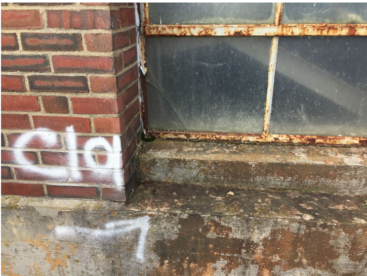
Asbestos caulk on Units 1&2 windows (Sample set C-01)
