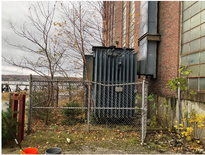
Northern exterior transformer cage.
