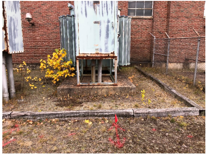
Southwestern exterior transformer cage.
