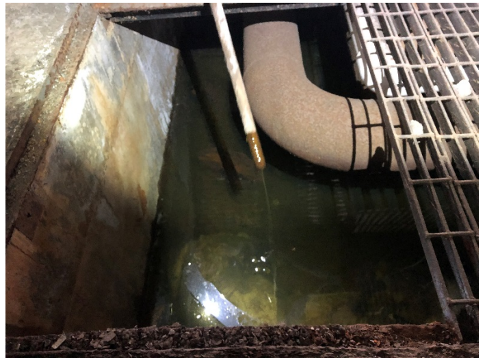
Tranformer oil release, Unit 5.
