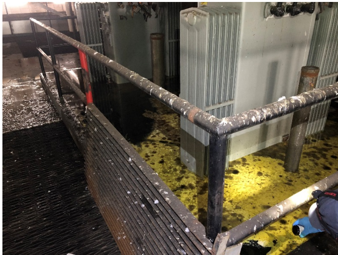
Transformer oil release, Unit 4.
