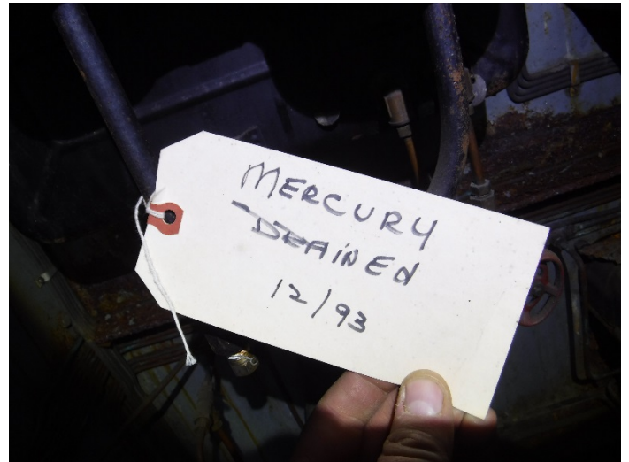
Tag within cabinets depicted on photo to the left.
