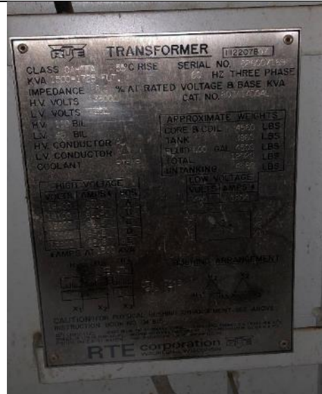
Photo 2: Transformer Information Plate.
