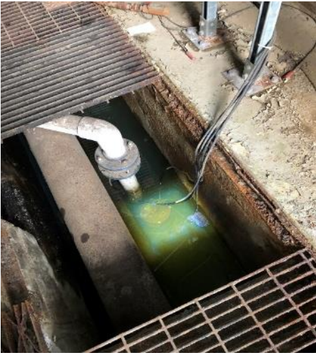
Photo 7: Oily water in trench drain system adjacent to leaking transformer.
