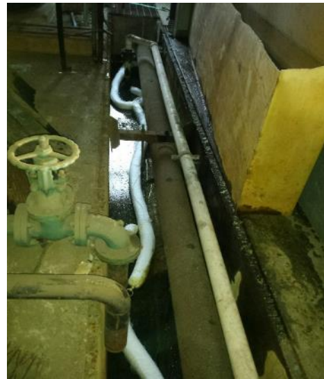
Photo 16: Trench drain with oily water prior to water removal and cleaning.
