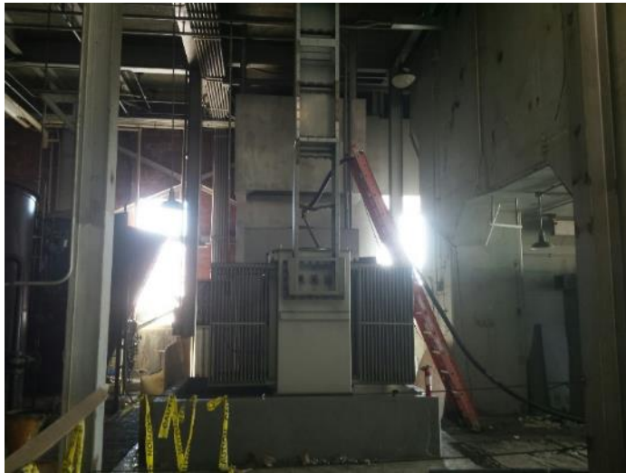
Photo 1: Unit #5 electrical transformer, prior to removal, looking east.
