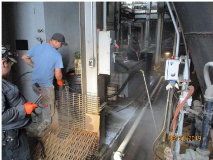
Photo 23: Power washing floor area adjacent to electrical transformer.
