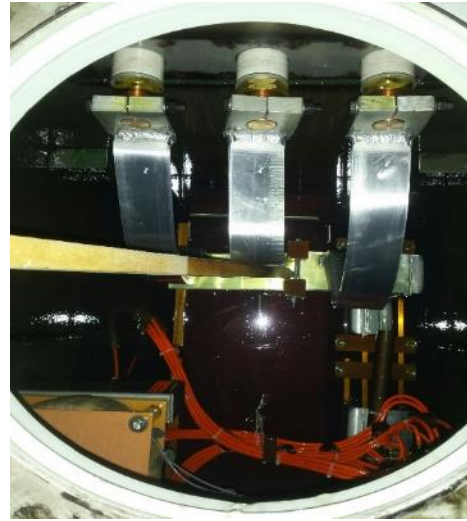
Photo 8: Interior of electrical transformer (looking down) prior to draining oil.
