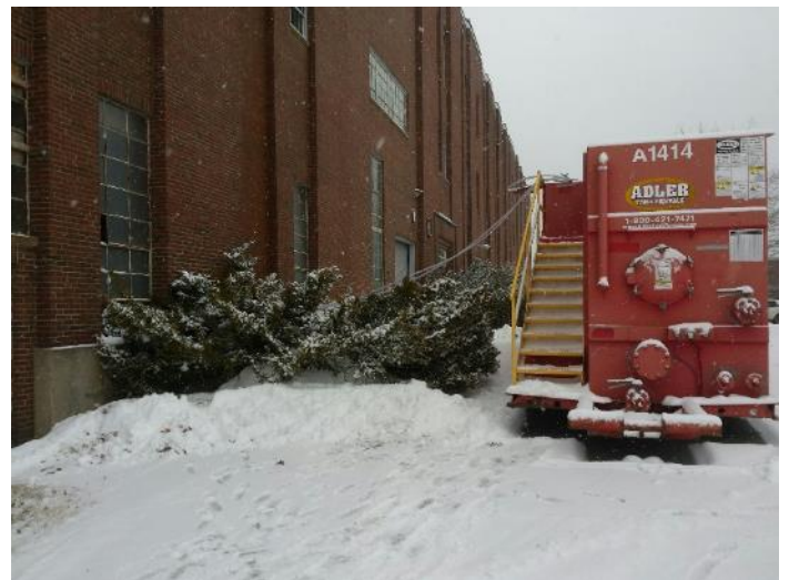
Photo 18: Frac tank for storage of treated water.
