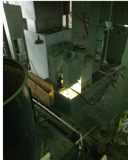
Photo 4: Transformer looking southeast from second floor.
