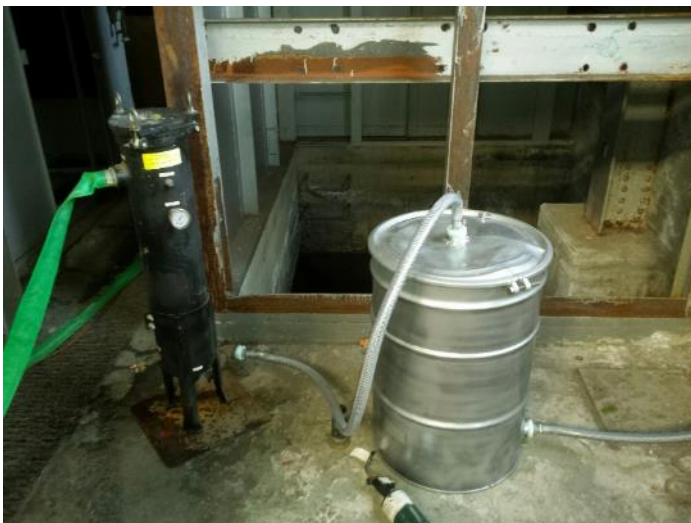
Photo 17: Bag filter and GAC drum for water treatment.
