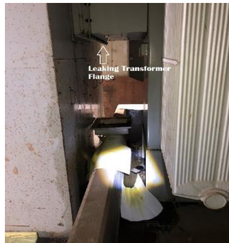
Photo 6: View of leaking flange on east side of transformer.
