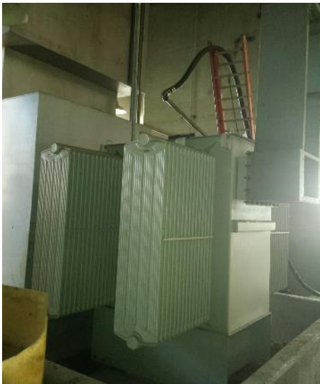
Photo 3: Electrical transformer looking southeast.
