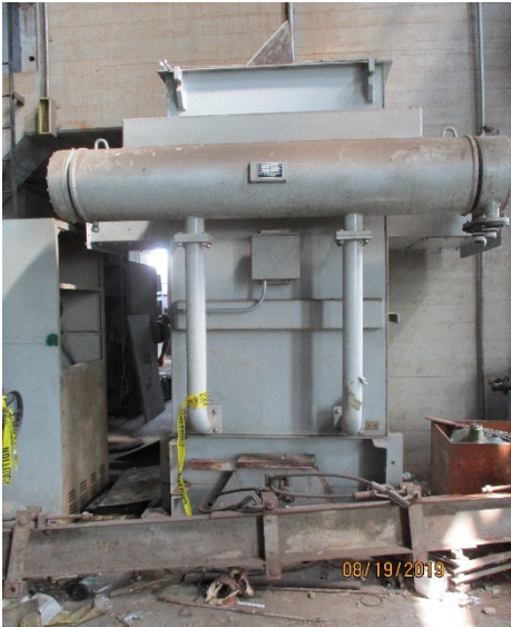
Photo 15: Transformer Serial number 51951.
