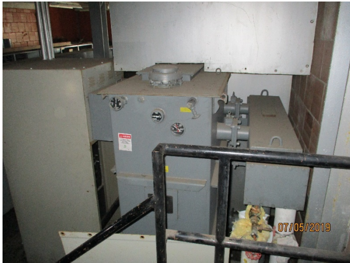
Photo 21: Transformer Serial Number 50541.
