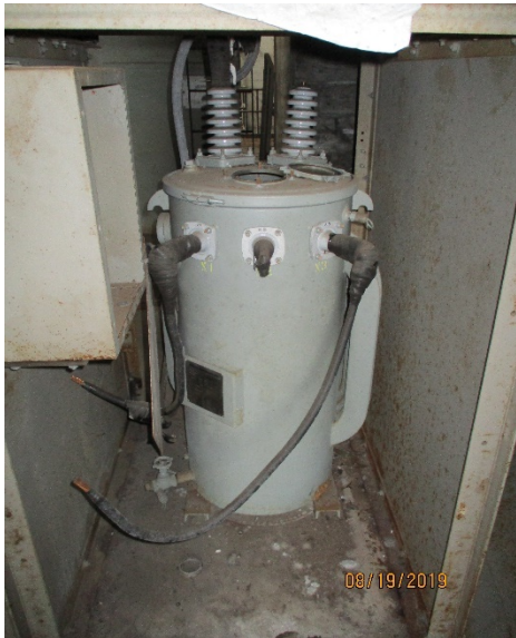
Photo 19: Transformer Serial Number 51337.
