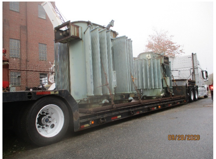
Photo 6: Loading Transformer No. 28477-1 for transport.
