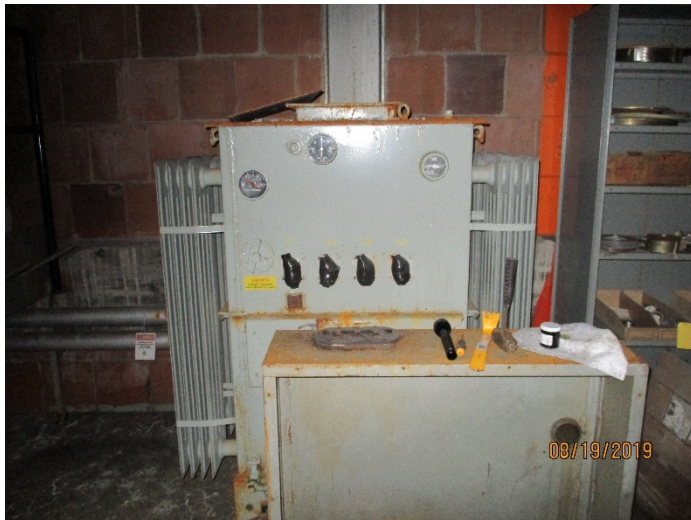
Photo 23: Transformer No I.D. Number.
