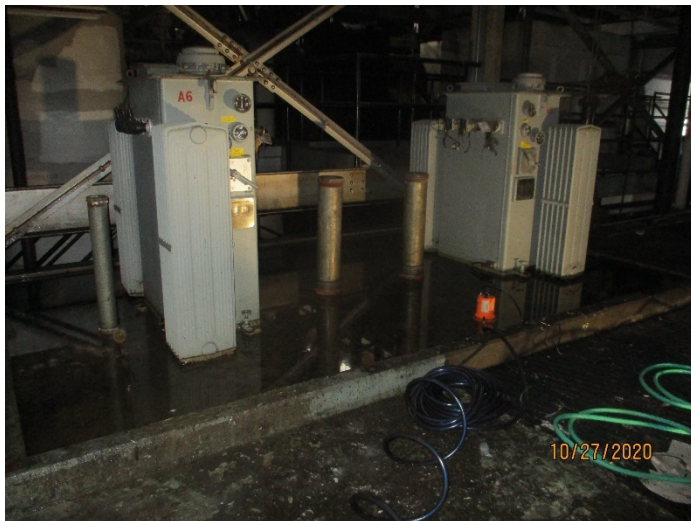
Photo 25: Transformer Serial Numbers 51334 and 51335 in spill containment structure.
