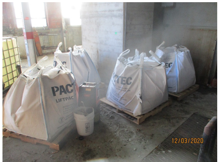
Photo 28: Totes of demolished concrete from spill containment structure, awaiting transport for disposal.
