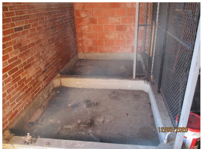
Photo 30: Location of Transformer Serial Numbers 516107 and 516678 following removal.
