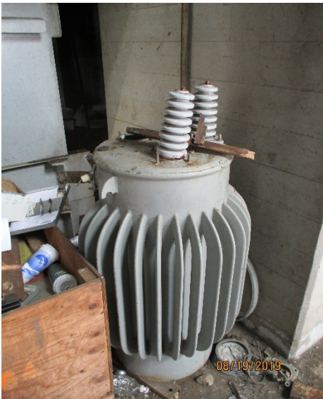
Photo 17: Transformer Serial Number 51336.
