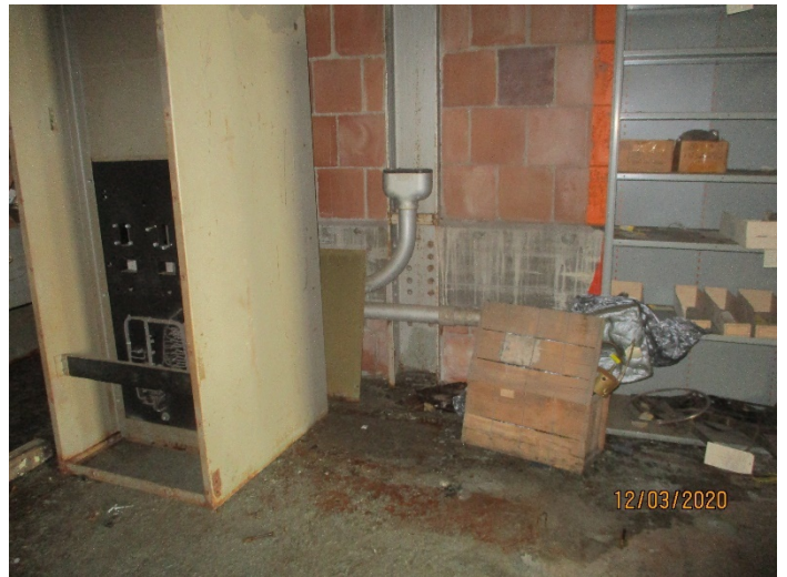
Photo 24: Location of Transformer No I.D. Number, following removal.
