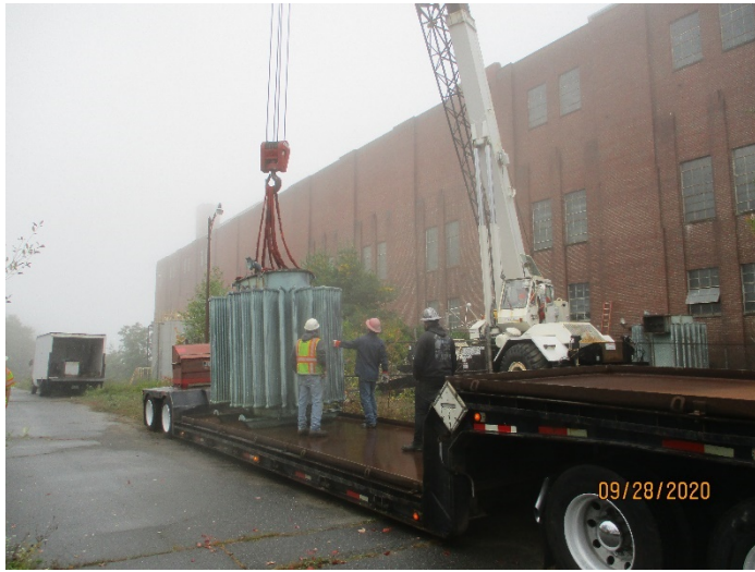
Photo 3: Loading Transformer No. 28479-1 for transport.
