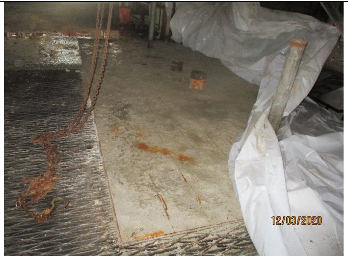
Photo 26: Spill containment structure following removal of Transformer Serial Numbers 51334 and 51335, oily water, and concrete.
