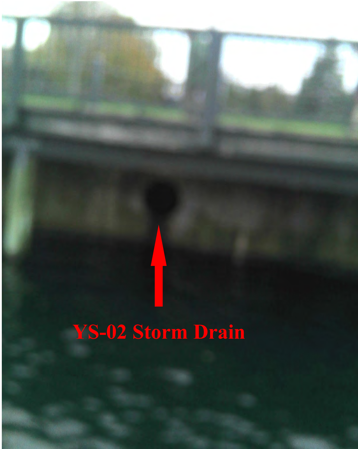
Photograph YS-02. View of the Parking Lot Storm Drain at Location YS-02 in the General Vicinity of the Yachting Solutions Marina Basin. Photographer Bud Brown, ECO-ANALYSTS, INC. November 2, 2017.
