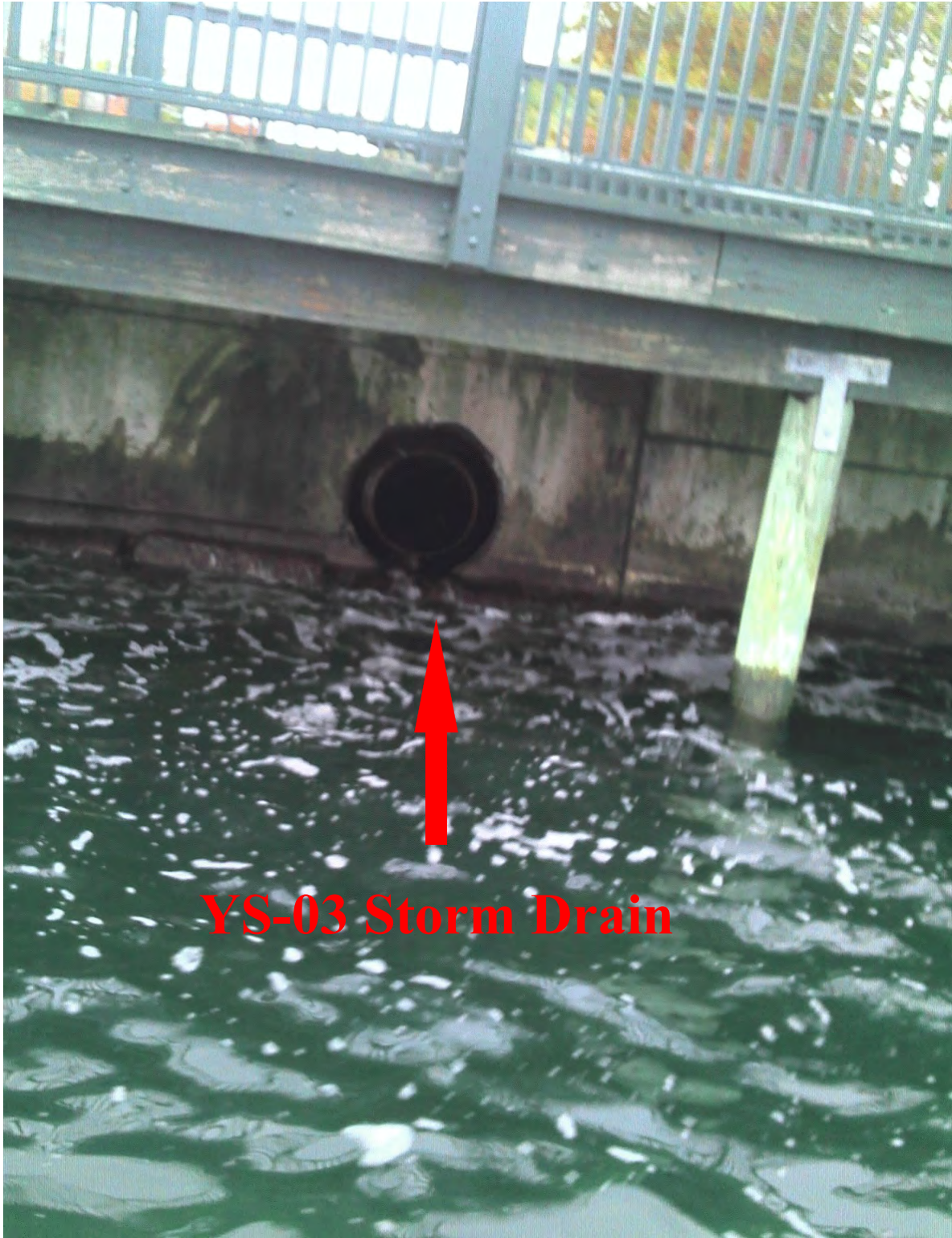
Photograph YS-03 View of the Parking Lot Storm Drain at Location YS-03 in the General Vicinity of the Yachting Solutions Marina Basin. Photographer Bud Brown, ECO-ANALYSTS, INC. November 2, 2017.
