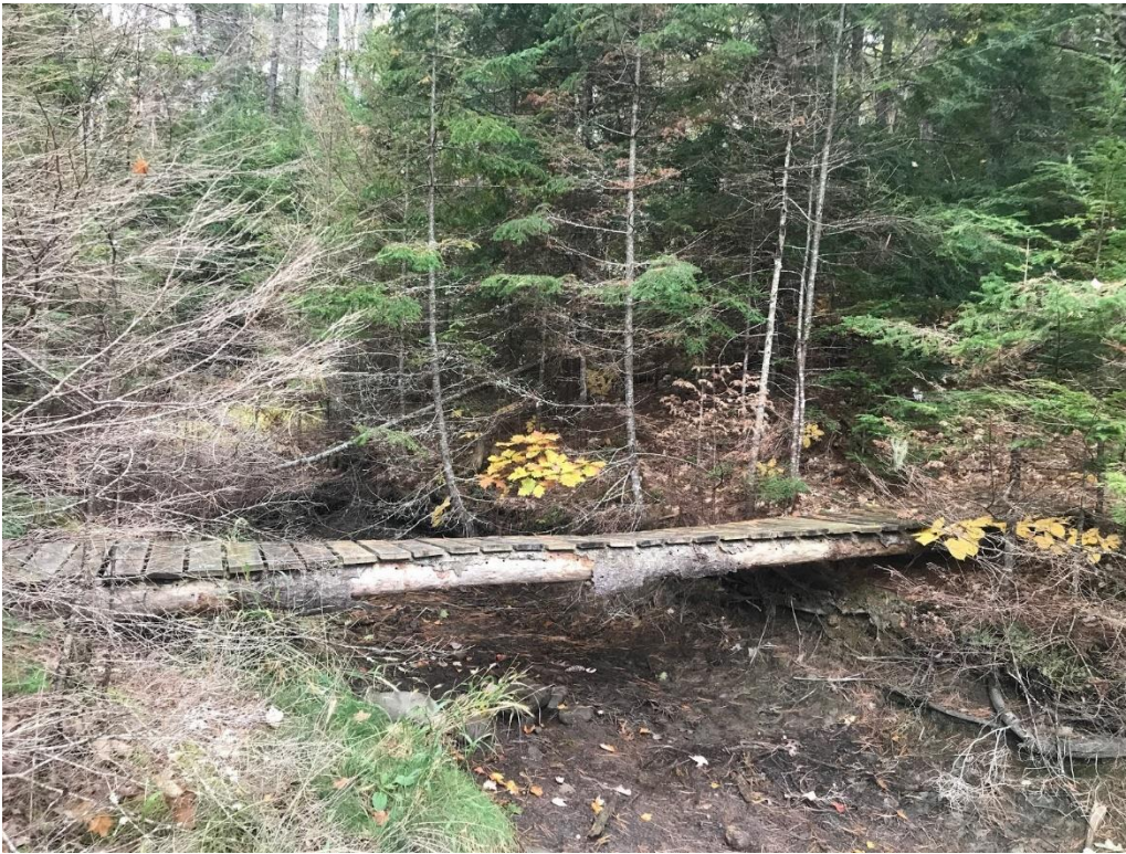
Photo 34: Bolen - unpermitted bridge structure over and adjacent to wetland
