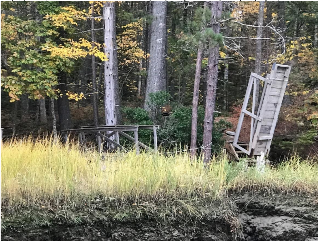
Photo 17: Lifted wooden dock/pier/floats with permanent concrete piers below HAT - (formerly Bill Mook) - Now Leah Sprague - commenter
