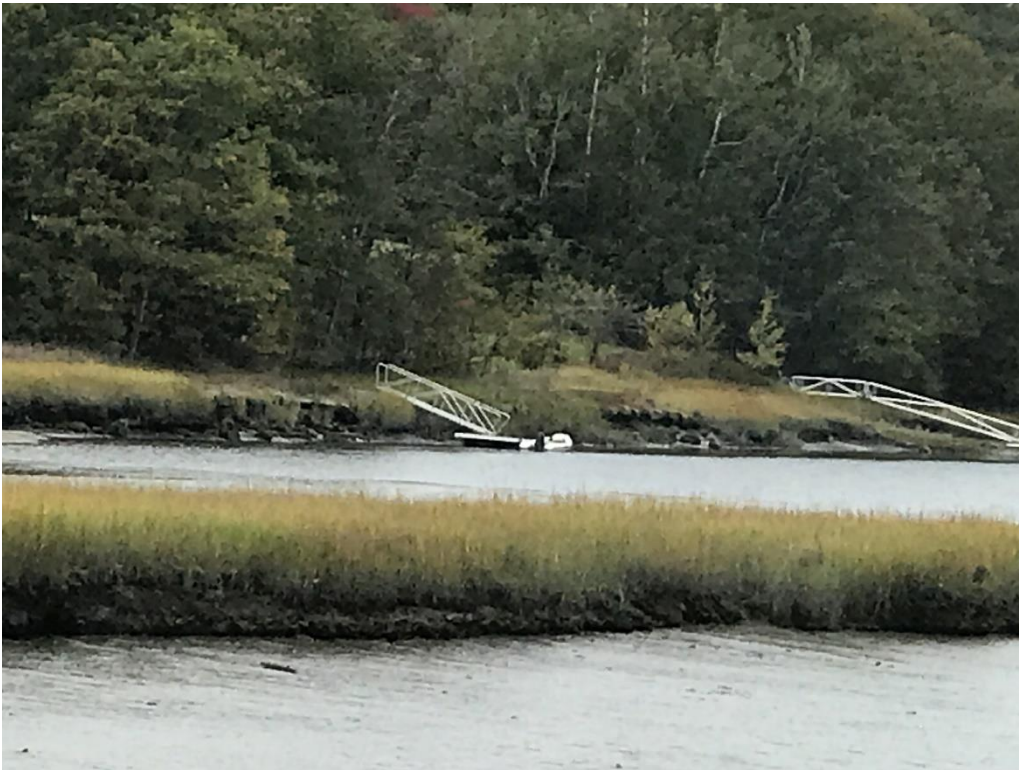
Photo 72: Whittemore - Dock w/ upland piles, ramp, float and ~16' zodiac center console (left hand) – Whittemore
