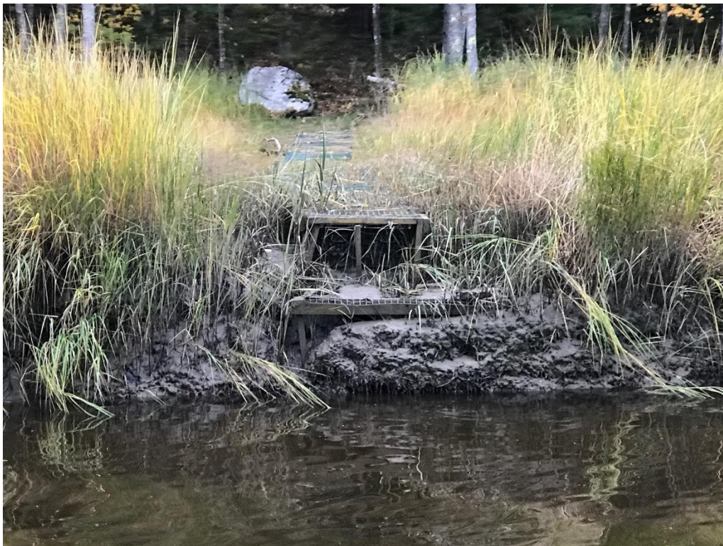
Photo 13: Steve Chef - walkway mowed/cut through saltmarsh (permanent structure laid into marsh grass as walkway & steps) - commenter, likely unpermitted
