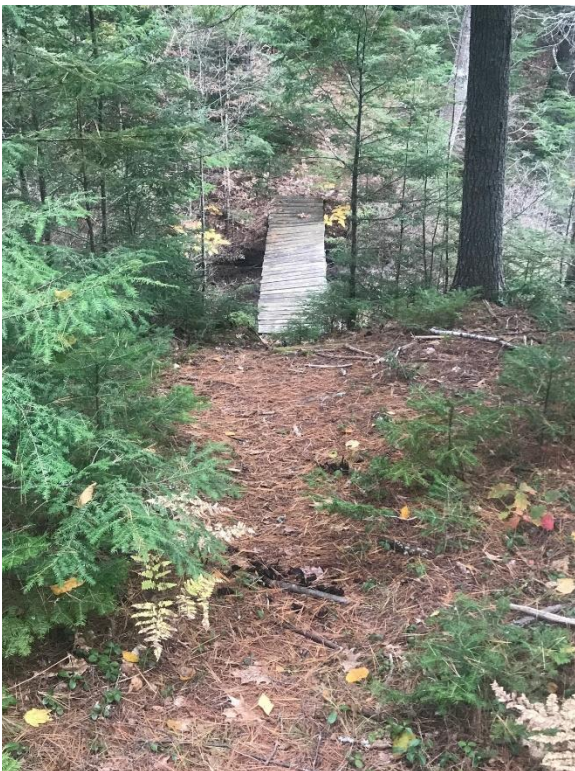
Photo 33: Bolen - unpermitted bridge structure over and adjacent to wetland
