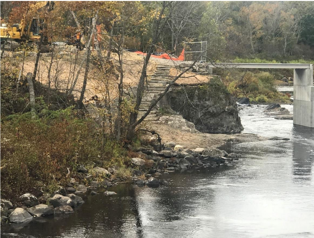
Photo 6: Head Tide Dam, views up and down river, and parking, and stairs. NOT YET COMPLETE
