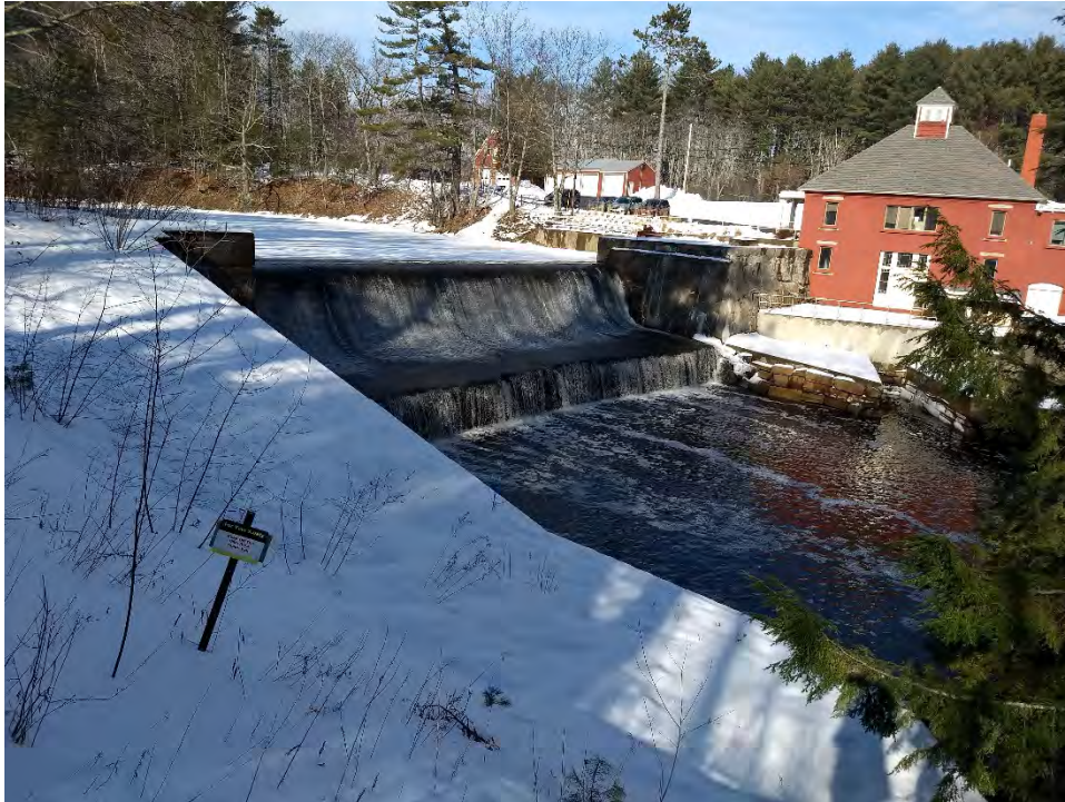
Photo No. 21 – Lower Dam – looking towards left abutment. Note cracking with efflorescence on left abutment.
