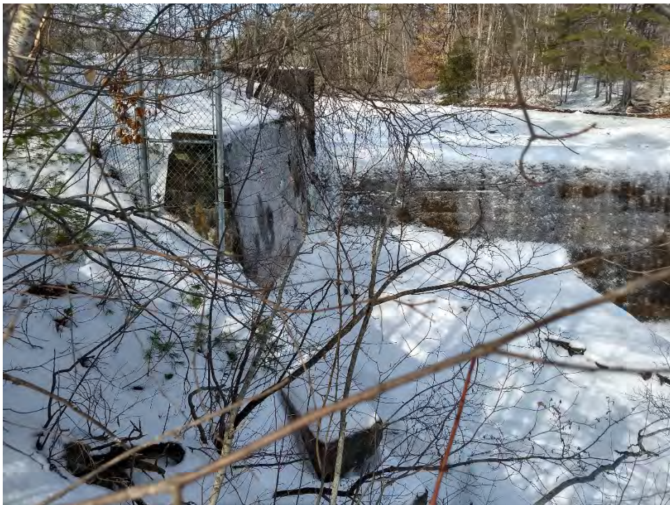
Photo No. 12 – Upper Dam – Right downstream side of spillway and downstream training wall.
