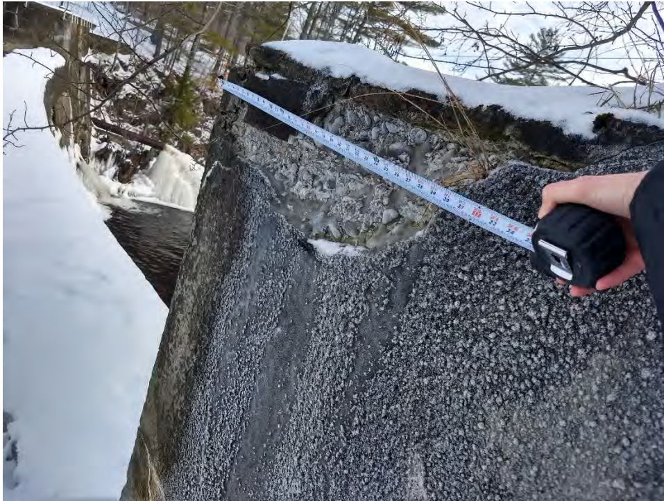
Photo No. 10 – Upper Dam – Upstream side of right abutment retaining wall. Note spalling concrete.
