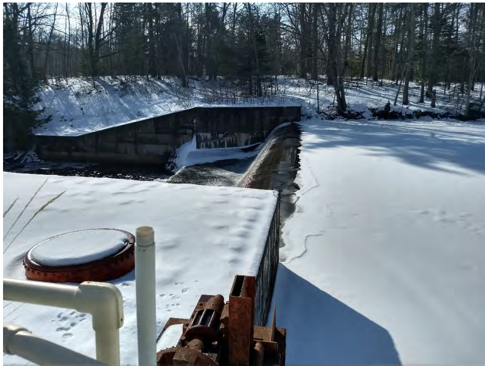
Photo No. 18 – Lower Dam – looking right. Note cracking with efflorescence on right abutment.
