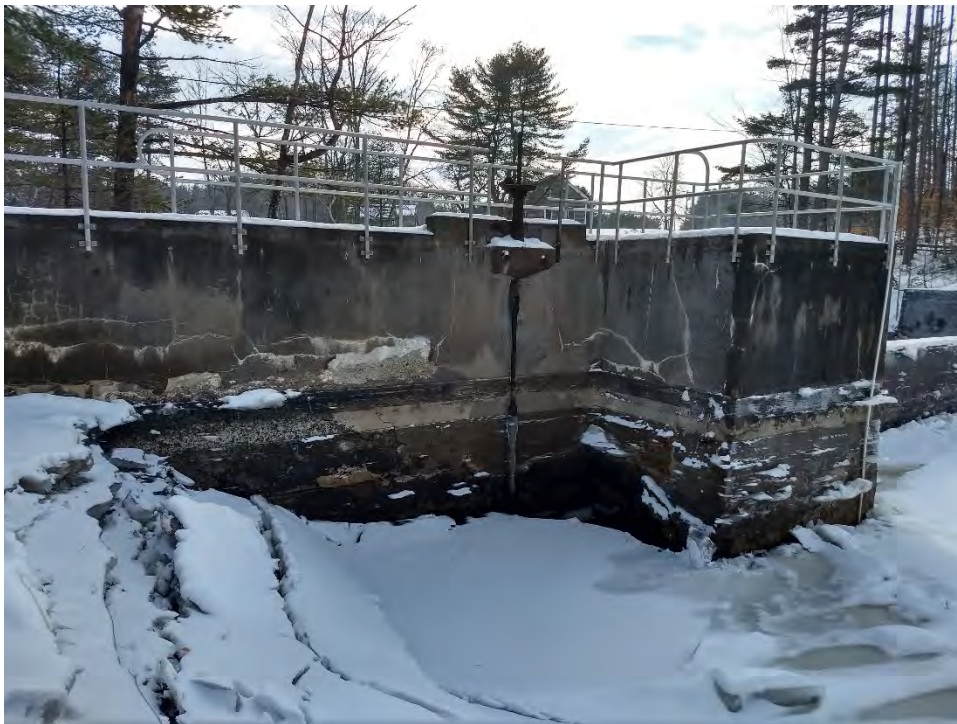
Photo No. 6 – Upper Dam – Upstream side of left abutment. Note 18" gate stem and cracking and spalling concrete.
