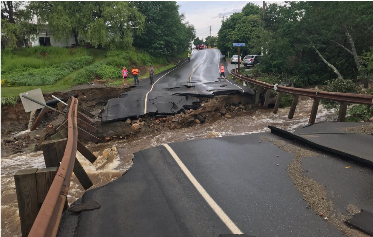
Road damage from June 2021 storm in Birch Harbor. Photo: Dale Church Thanks to Bill Zoellick for helping to prepare this summary.
