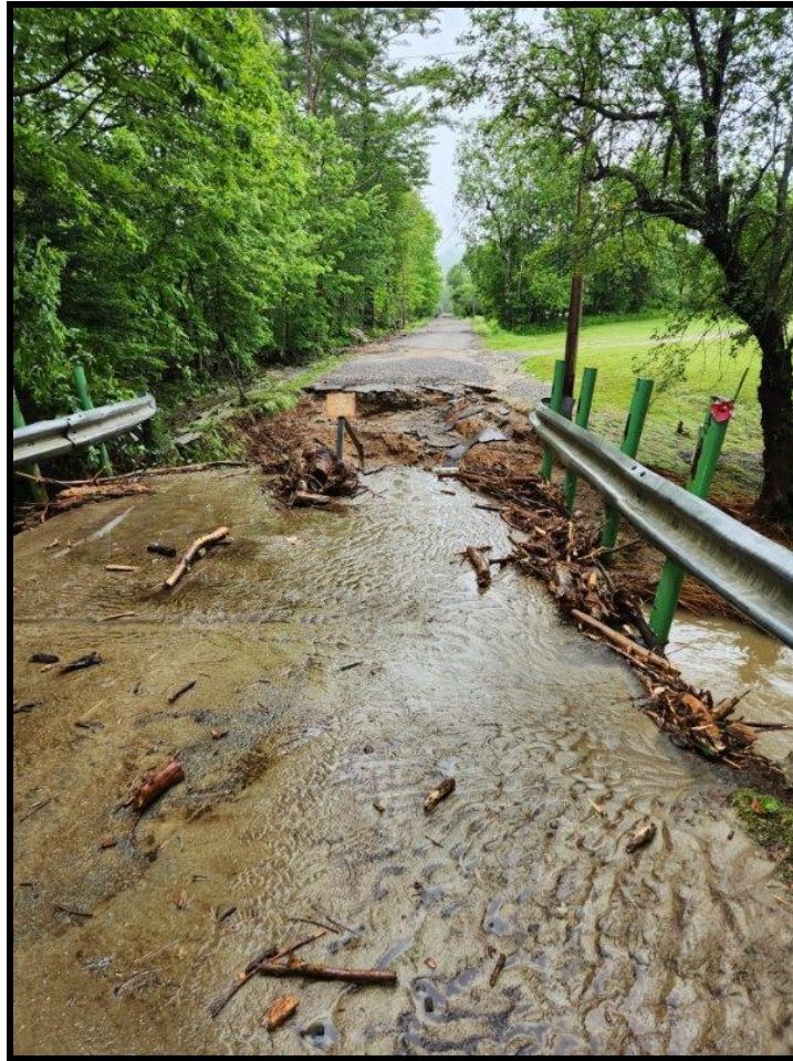
Jun 26, 2023 damage on Wyman Hill Rd in Andover, ME
