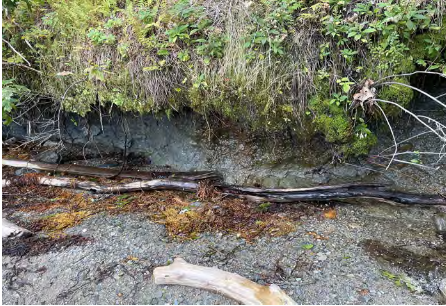
Photo 5. Steep eroding upland bank at Sears Island. September 2023.
